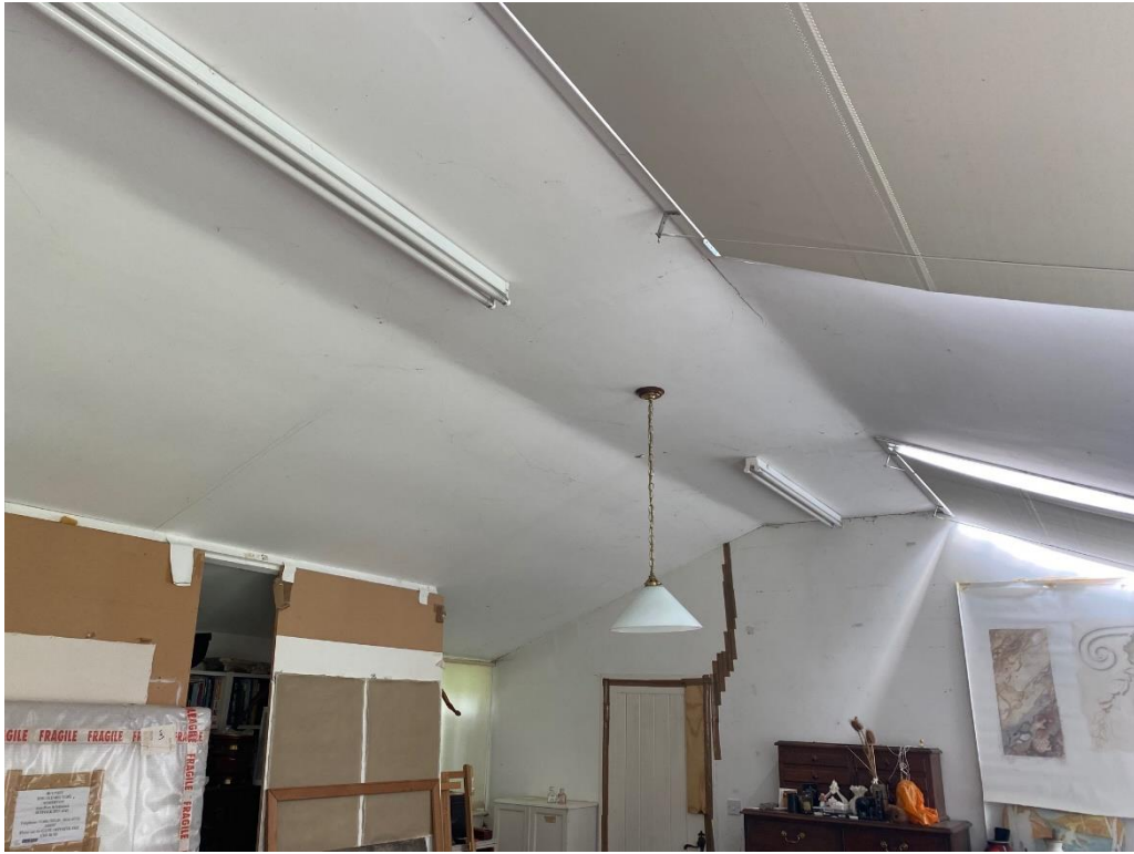
Building 1 – internal view showing location of cracking to partition wall
