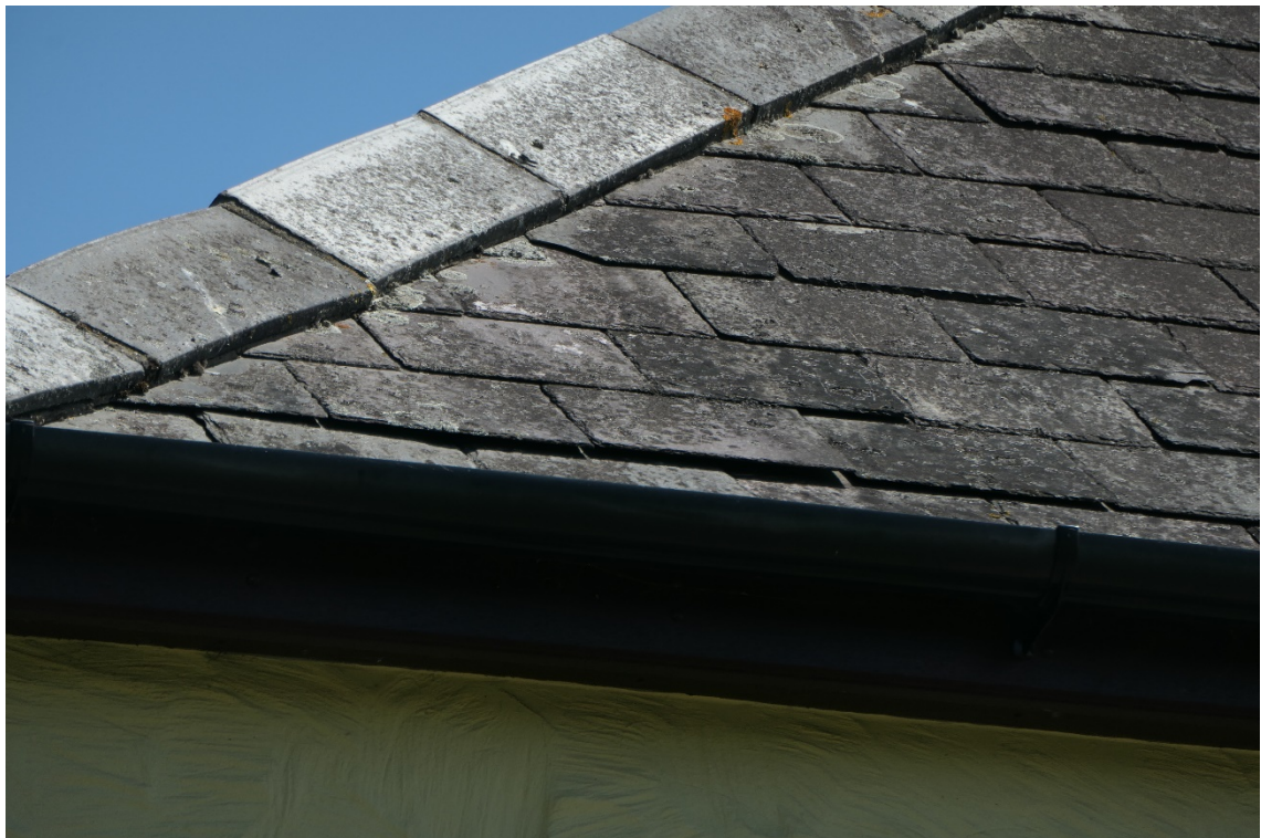
Photo 7 , lifted and distorted tiles on the northwest corner of the building provides potential roosting feature and/or access point to the loft space.
