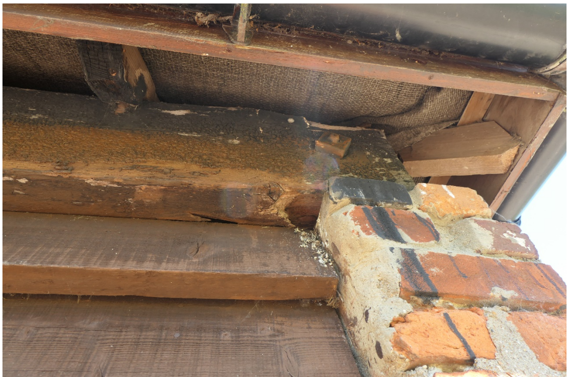
Photo 10 , gaps beneath weatherboard, between timber and brick and in open eaves provide suitable roosting features and access points.
