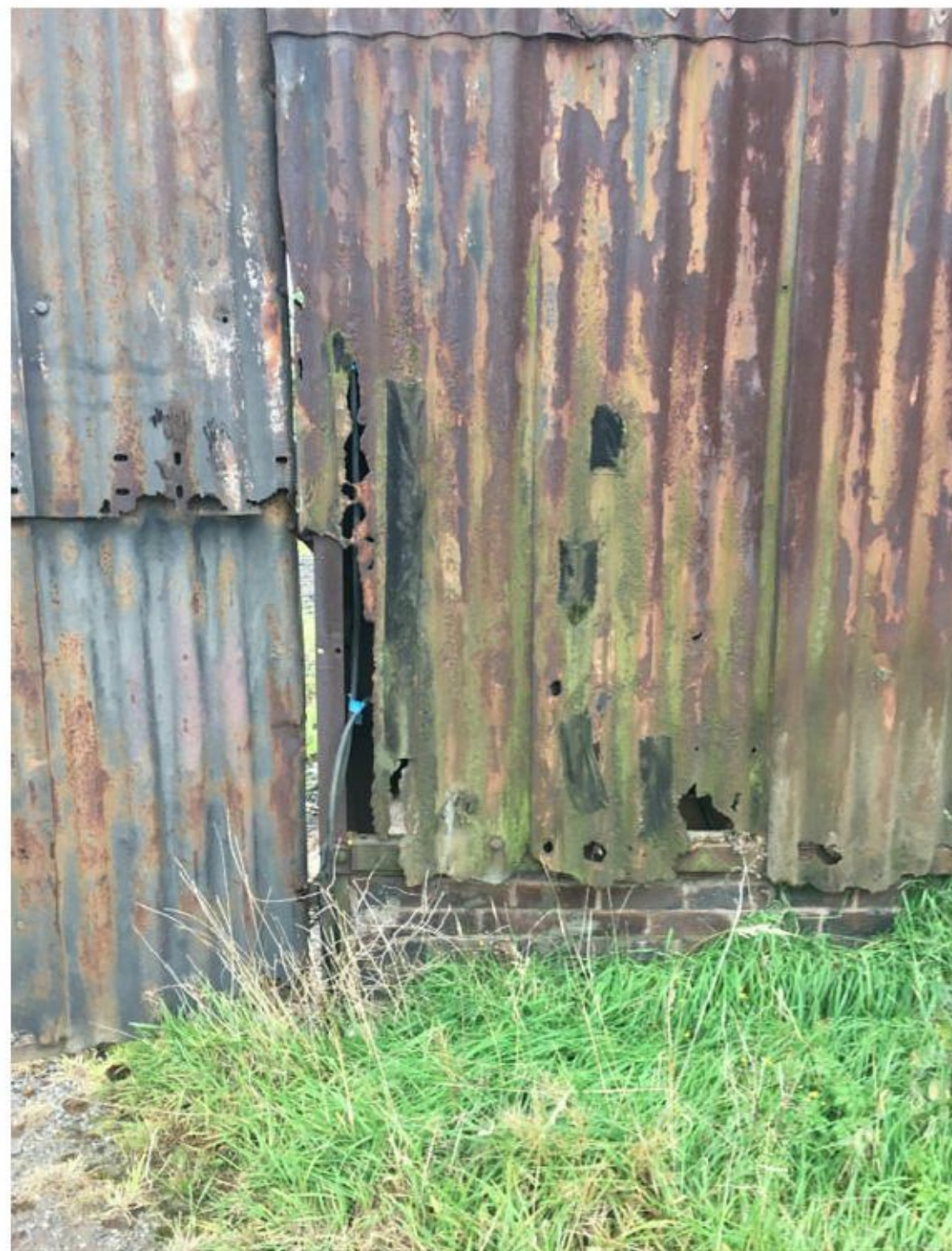
Figure 8: Metal cladding corrosion.
