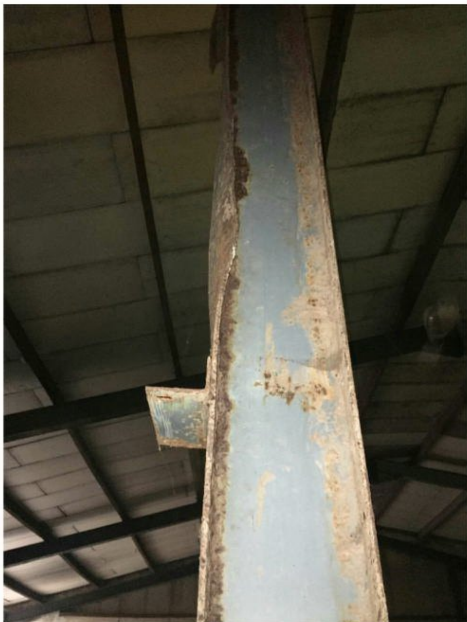
Figure 4: Flange distortion to internal column.
