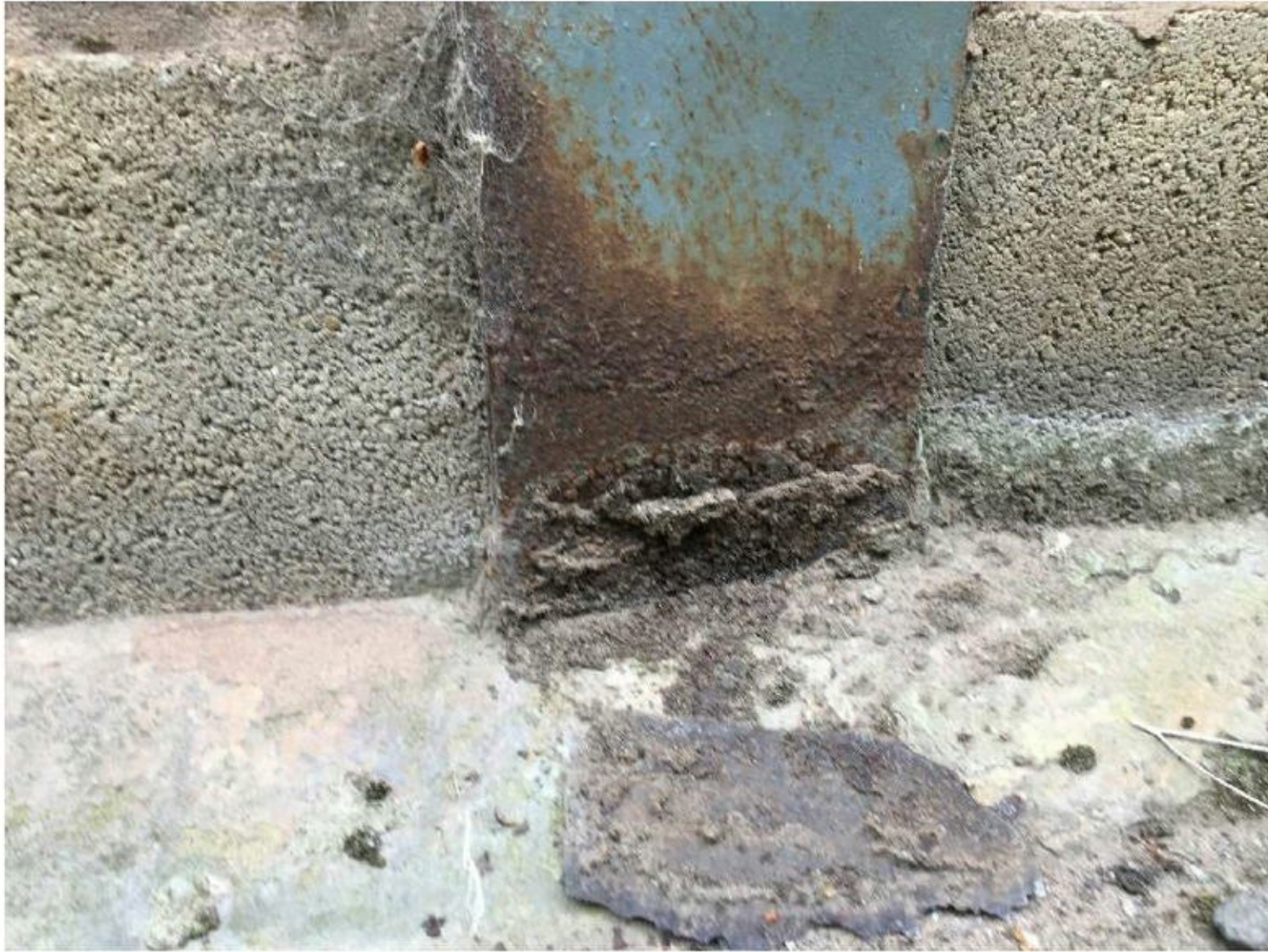
Figure 7: External column corrosion.
