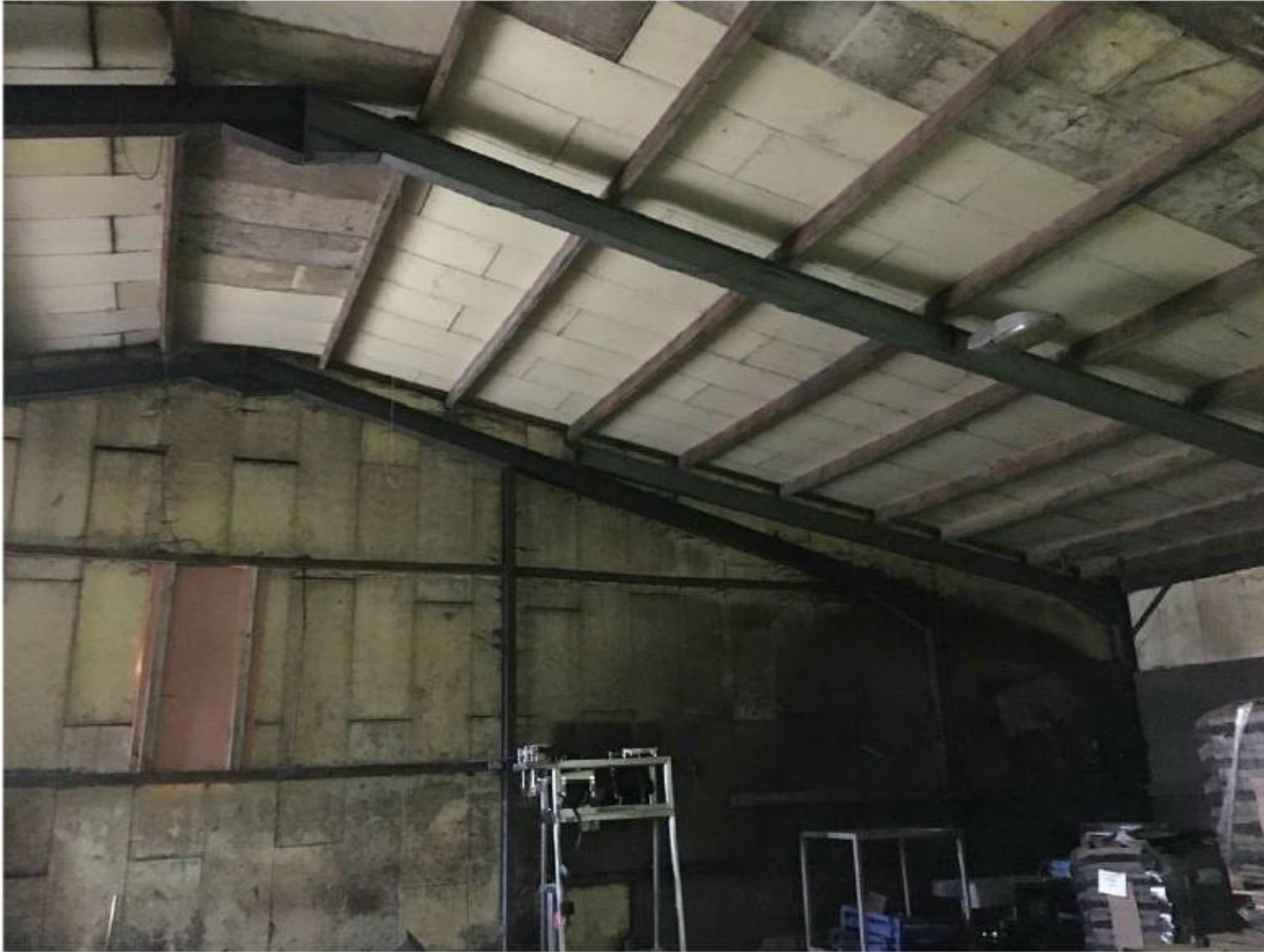
Figure 1: Differing paint specification noted to both sides of the portal frame.
