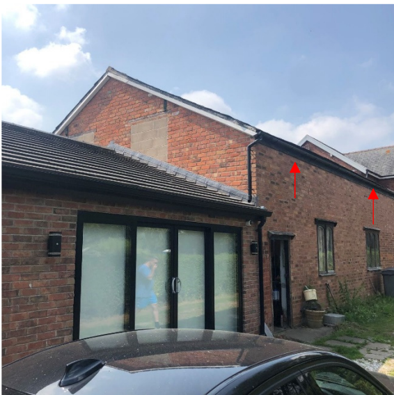
Photograph 3: PRF3 gaps between wooden fascia board and brick wall on north elevation.
