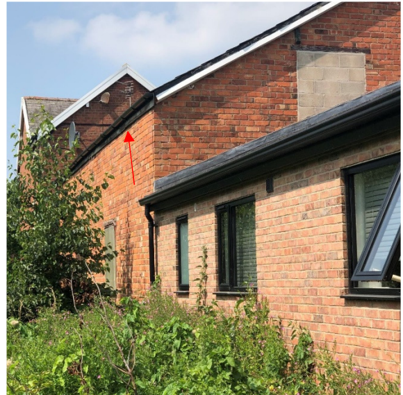
Photograph 4: PRF4 gaps between wooden fascia board and brick wall on south elevation.
