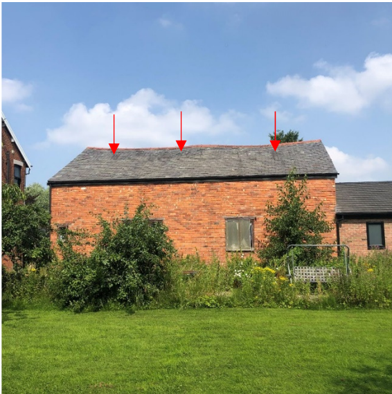
Photograph 2: PRF2 gaps on the south roof pitch where slates have become dislodged.
