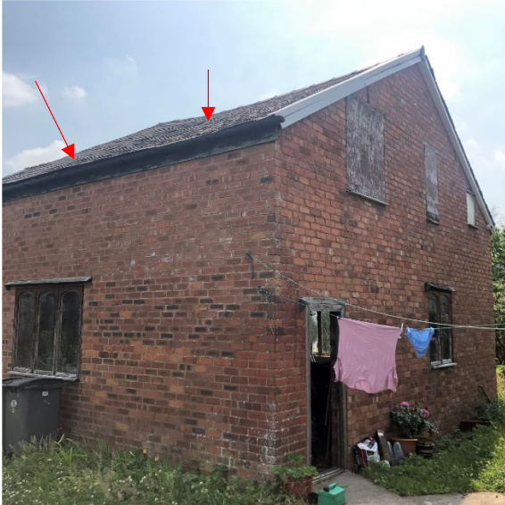
Photograph 1: PRF1 gaps on the north roof pitch where slates have become dislodged.
