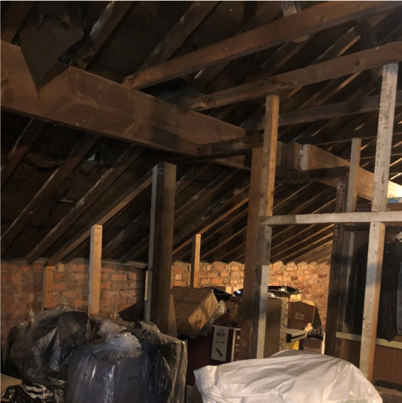
Photograph 7: View of the north internal roof pitch. Gaps observed in felt and slates allowing daylight through.
