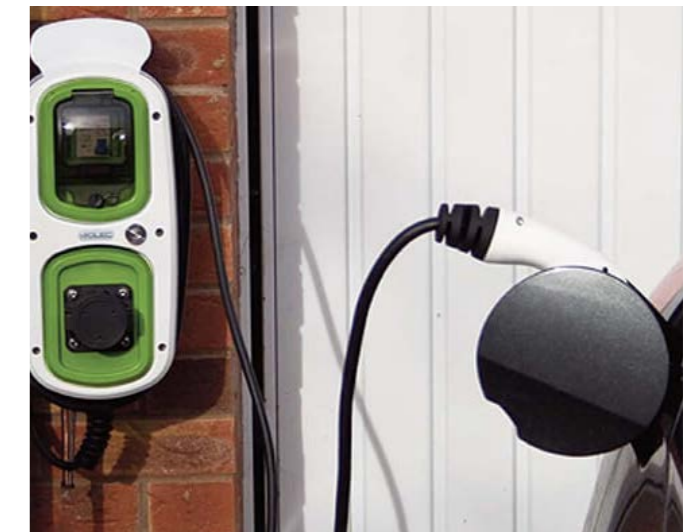
electric car charging points next to all parking spaces
