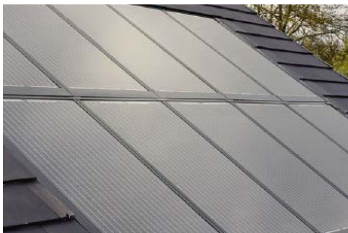
PV array integrated into roof design
