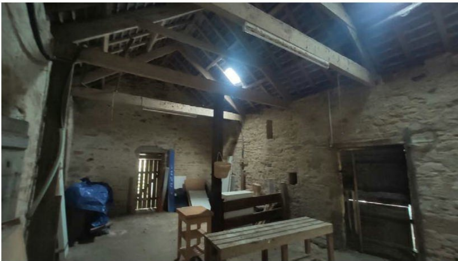
Photograph: 6 Showing an internal view of the stone built thrashing barn in the north west of the site. This will be retained as part of the development.
