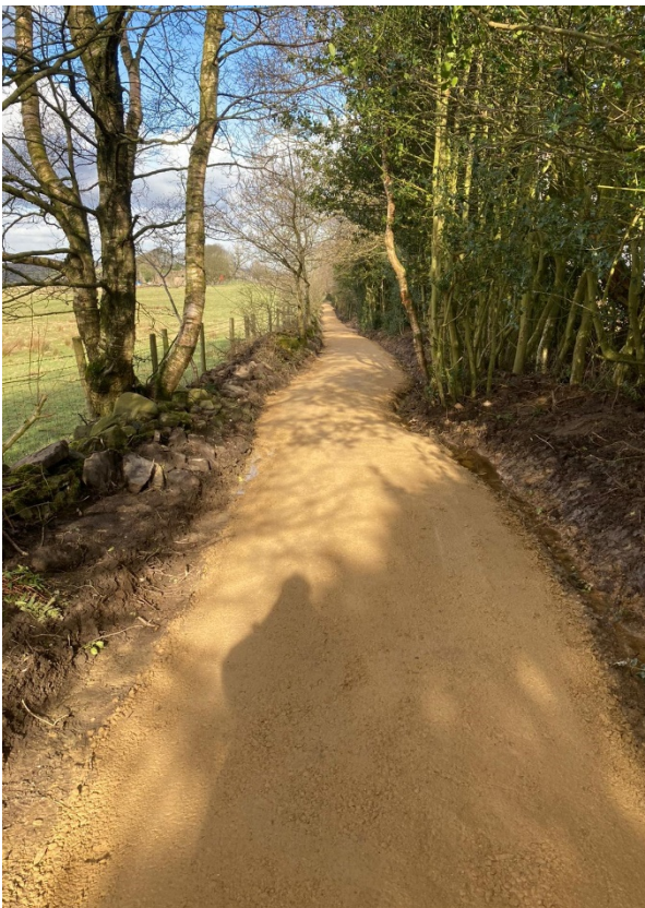
Plate 2 - A view of a path laid using the same methodology and materials on another National Trust property seen immediate after laying.
