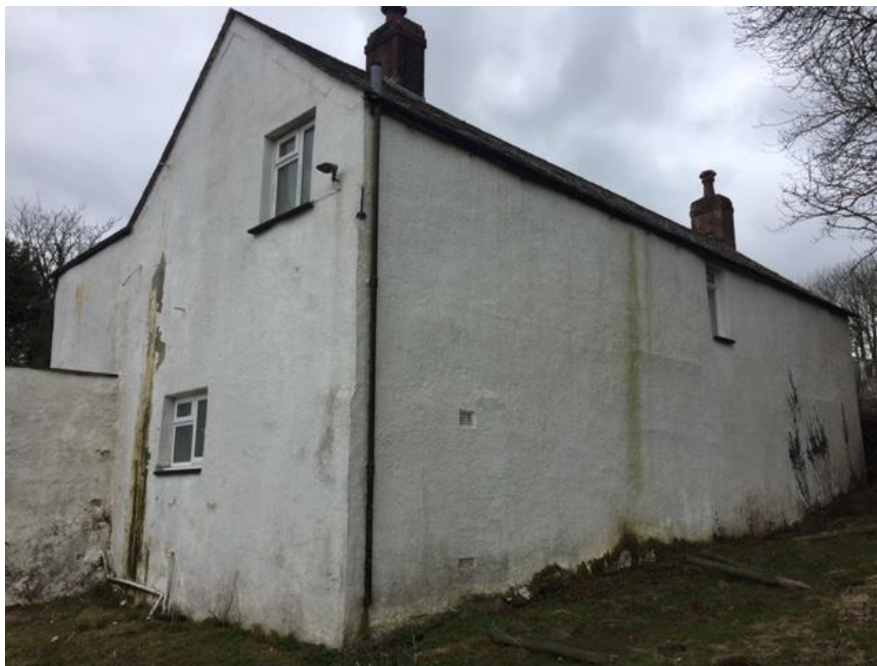
Fig. 6: The North elevation of the main dwelling, where rising damp can be seen on the rendered external stone walls. Image shows the land falling from West to East to the right of shot, seen against base of northern elevation.
