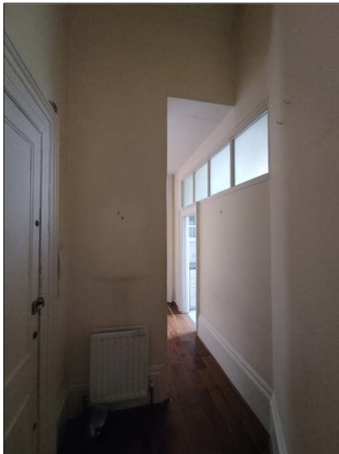
View C - View down entrance corridor. New dropped ceiling beyond to be removed & ceiling level to be taken back to original and original room depth to be re-instated. Existing non loadbearing wall with clerestorey to be replaced with new. New glass clerestorey to run from top of new door opening to underside of ceiling allowing original volume and corning to be revealed
