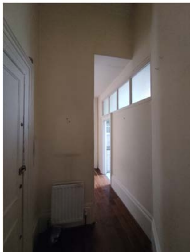
View C - View down entrance corridor. New dropped ceiling beyond to be removed & ceiling level to be taken back to original and original room depth to be re-instated. Existing non loadbearing wall with clerestory to be replaced with new. New glass clerestory to run from top of new door opening to underside of ceiling allowing original volume and cornicing to be revealed
