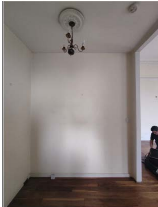
View A - Lobby area adjacent to living room and kitchen. New dropped ceiling to be removed & ceiling level to be taken back to original and original room depth to be re-instated
