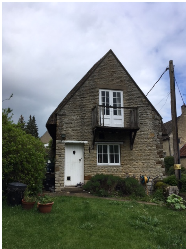
Fig 4. Existing derelict balcony in need of replacement
