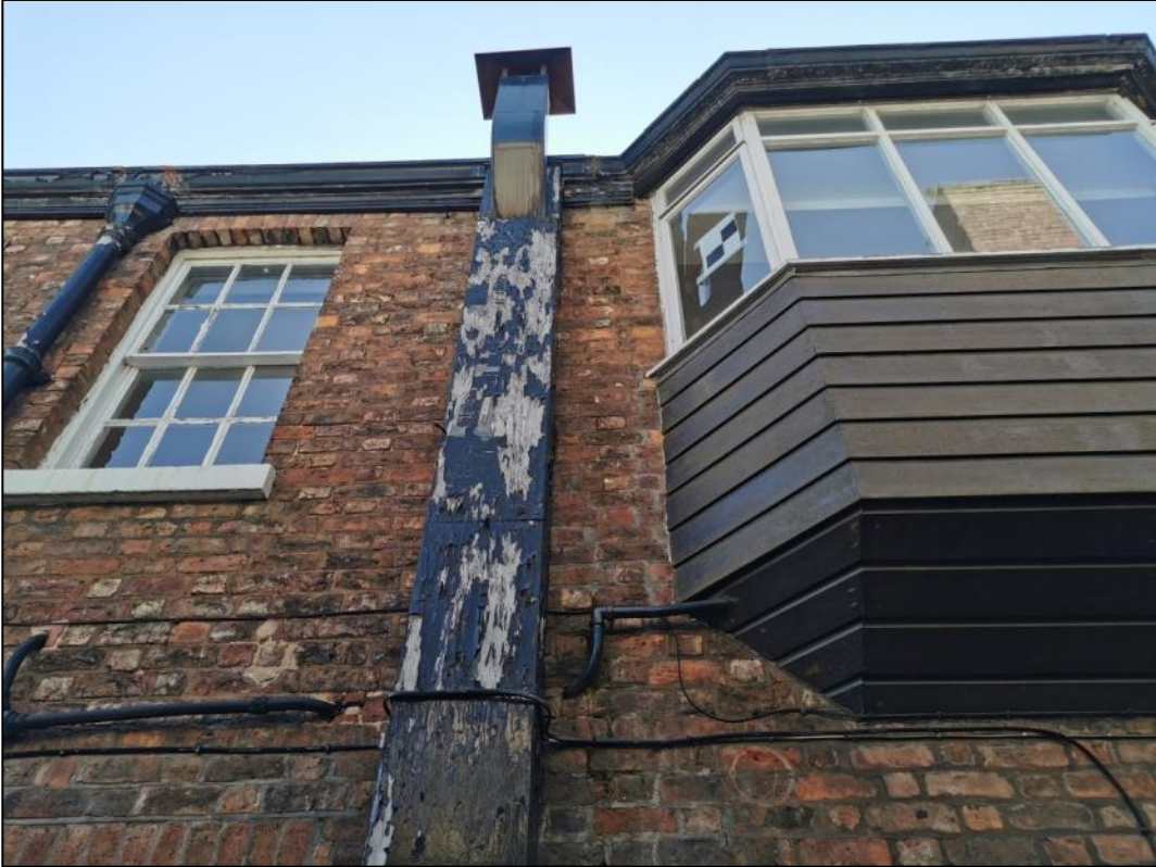
Plate 5 – Side with access road, west facing elevation brick segment - view of features
