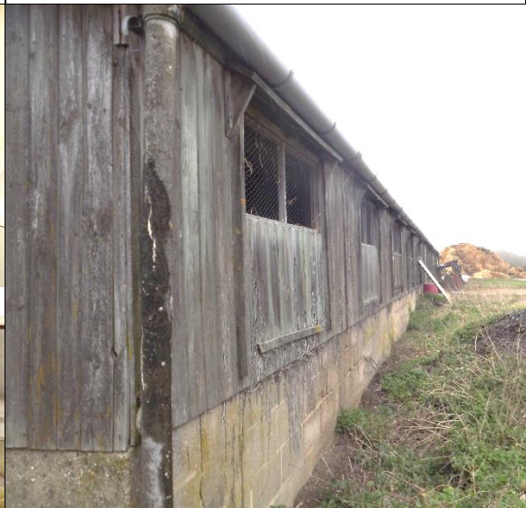
Bottom right: Additional access points through windows and example of the close-fitting external timber boards.
