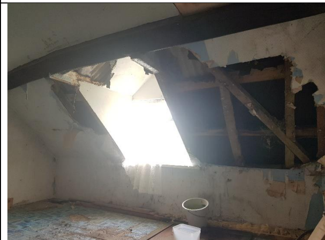
First floor of side extension. Ceiling failing in places.
