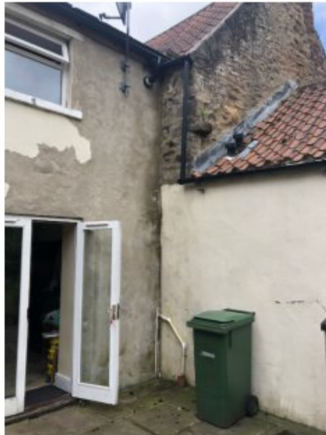
North west corner showing damp area from poor roof drainage
