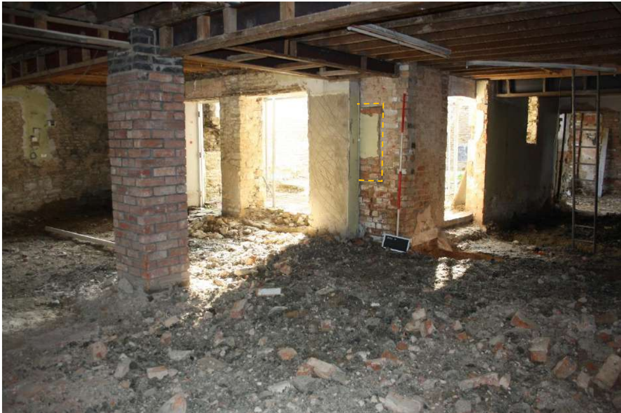
Plate 7: 3-4 looking southeast and showing bricked up window.
