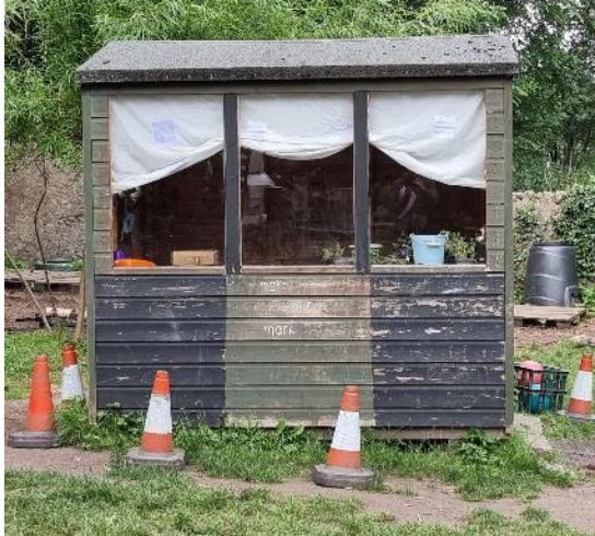
Photo 3. Potential roost feature – rotted roof at drain pipe.
