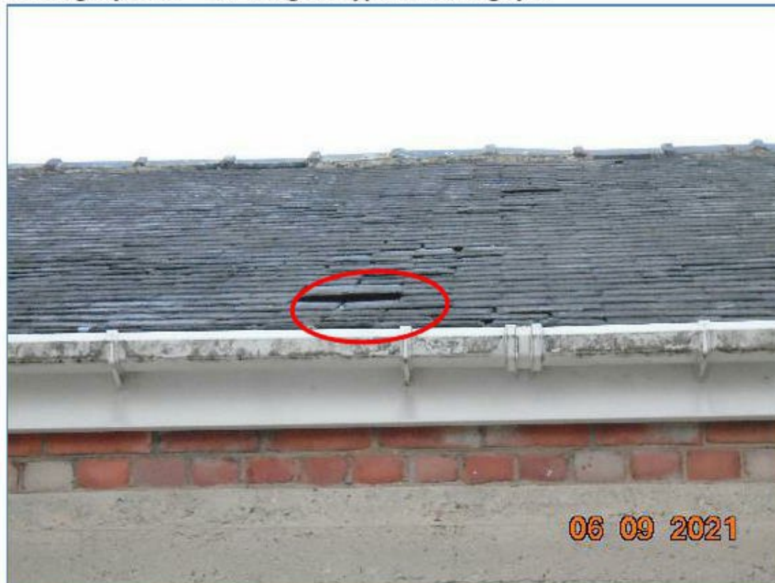
Photograph 15 – Building 1: Typical slate gaps.
