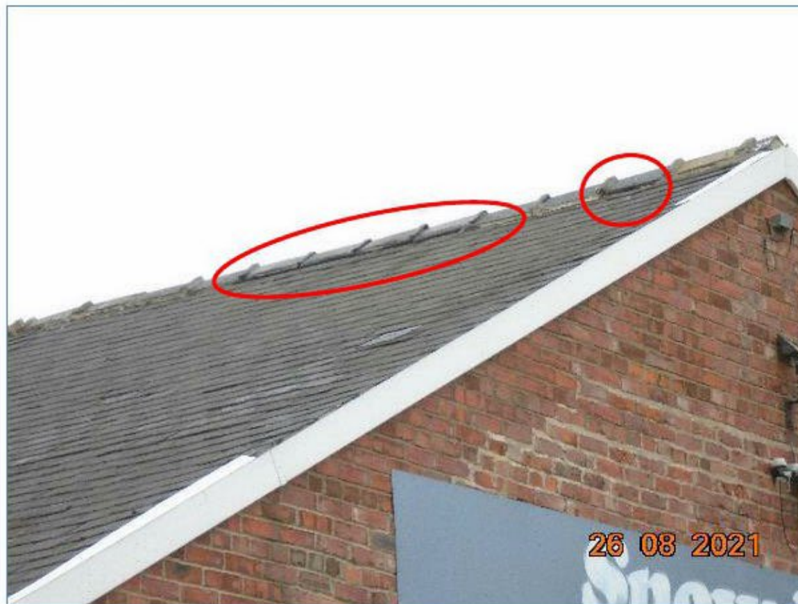
Photograph 13 – Building 1: Typical ridge gaps.
