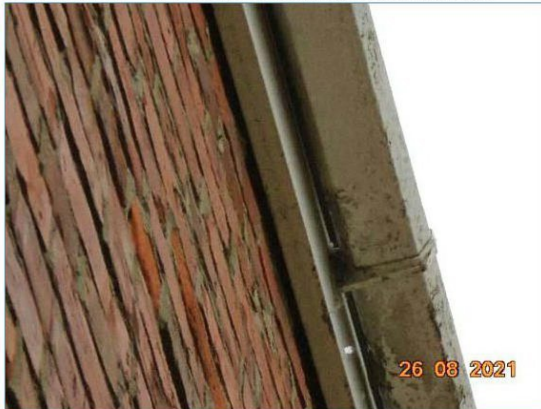
Photograph 14 – Building 1: Fascia gap to eastern elevation.
