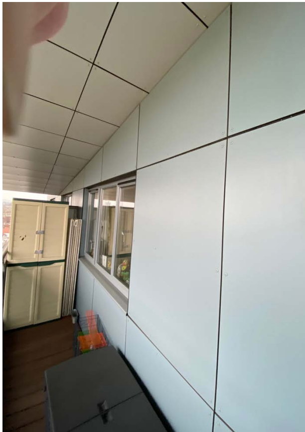
Top floor _ High Pressure Laminated Wall Panels to the Penthouse Level with direct interface to Soffit Overhang
