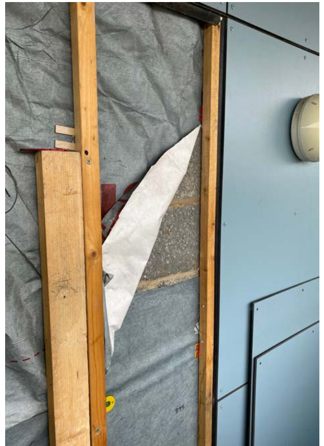
The HPL at the Penthouse Levels to the walling system with non-FR Tyvek membrane which adds to the risk of spread of fire across the facades.
