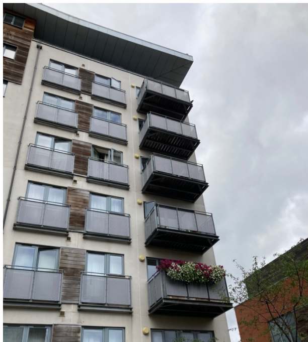
Projected Balconies and Juliette balconies _ showing the timber cladding and timber decking.
