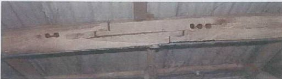
Scarf joint connecting the older frame to the C19th one. Note the holes for abandoned mortices.
