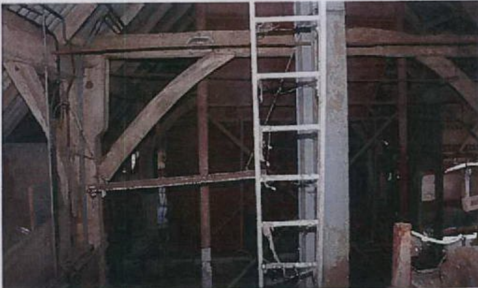
Detail of Truss 2 from the pre-dresser platform looking E. Note heavy jowl and spandrel.
