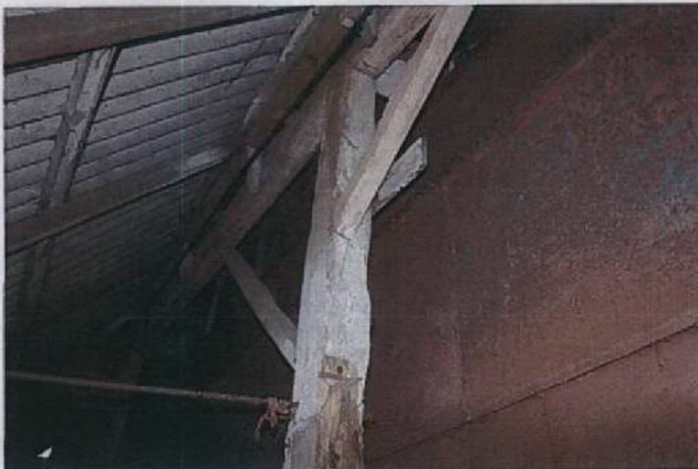
Detail of Truss 6. Note lack of jowl. Narrow braces and abandoned mortices.
