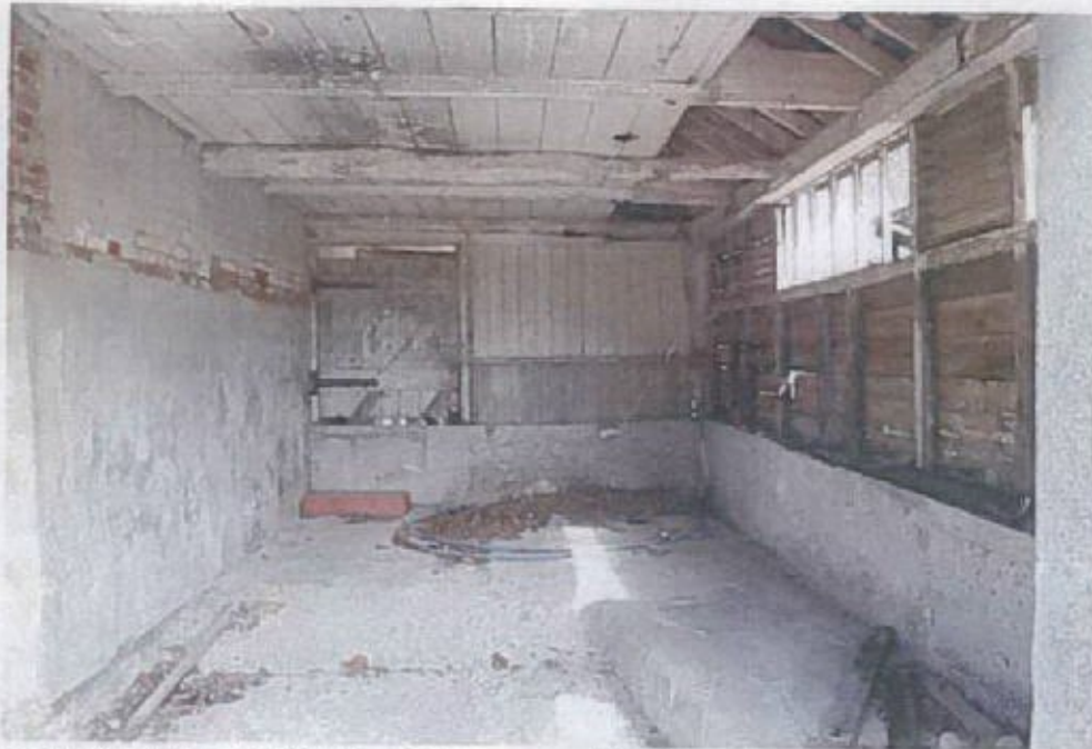
Looking N into the end of Shelter 3. This was a small milking parlour.
