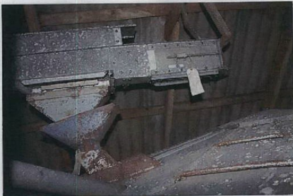
At the top the product could be diverted into the grain dryers or to the grain bins.
