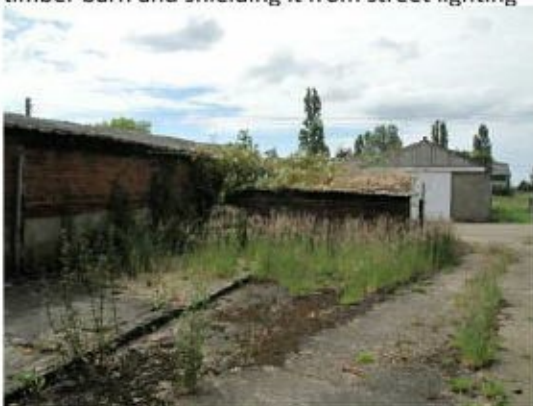
West elevation of the shelter sheds and the piggery covered in Russian vine
