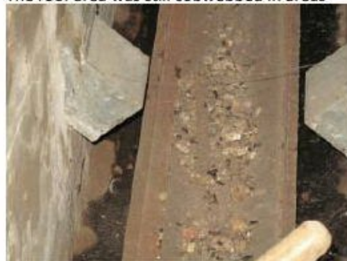
Rat droppings between the silos
