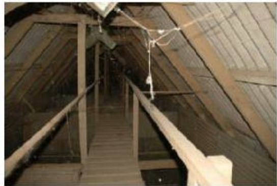
The roof area was still cobwebbed in areas
