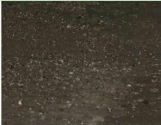
Pigeon guano was beginning to occur in quantity on areas of the floor
