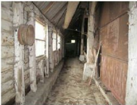
The interior of the barn was very dirty
