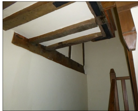
36 Remove staircase to 1st floor and reconfigure partitions to install kitchen & bathroom.
