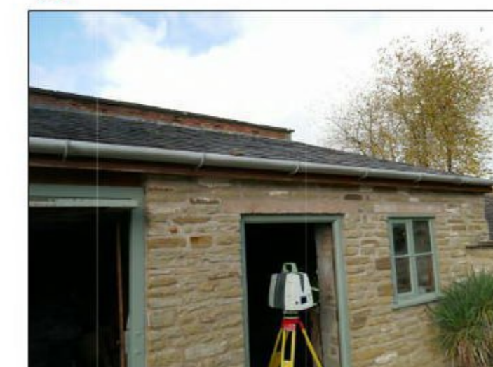
38 Remove existing garage roof to build new double pitched roof to accommodate Media Room.
