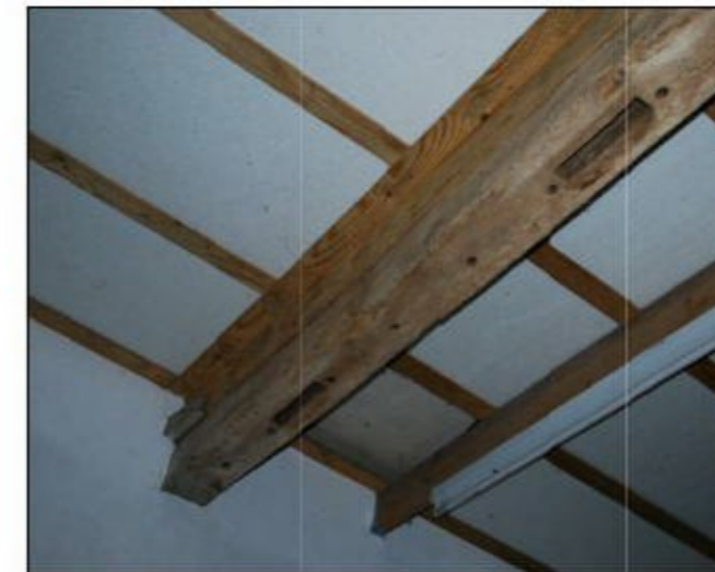
28 Remove modern false ceiling to rediscover double height and visible main trusses.
