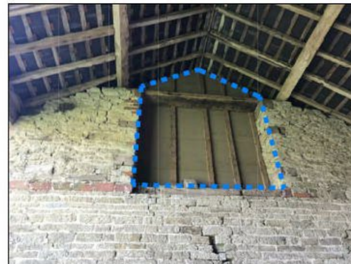
31 Remove modern lining to rediscover existing opening to be provided with new glazed joinery.
