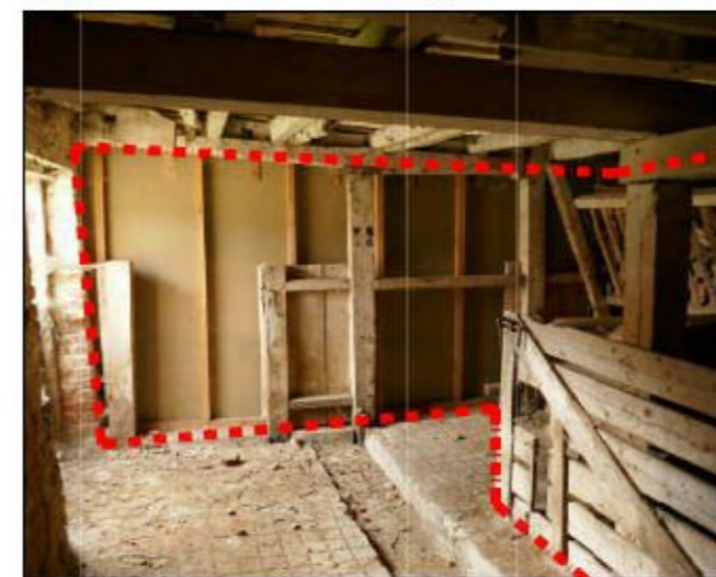
13 Remove stalls & modern dry lining to open up plan and allow more flexible use of GF.
