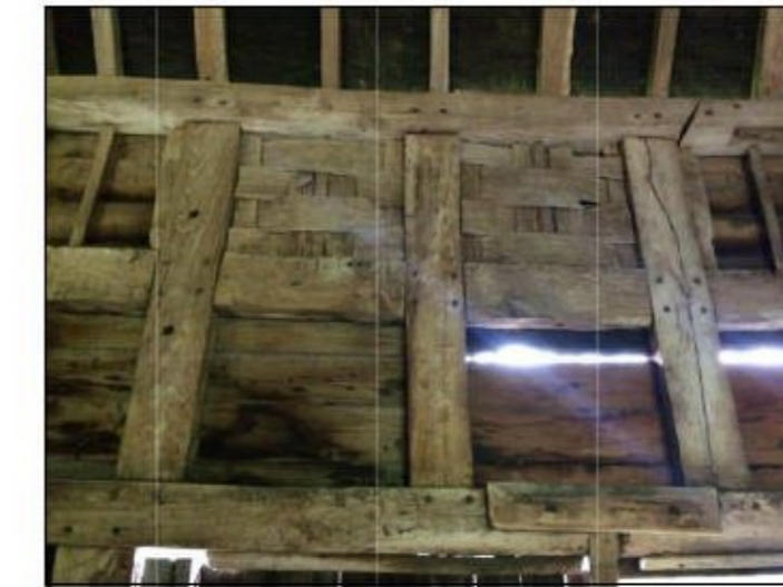
26 Remove modern timber boarding to reinstate woven panels within the existing timber framing.
