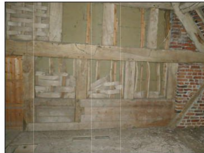
27 Remove modern lining to rediscover main truss & reinstate woven panels within the existing timber framing.
