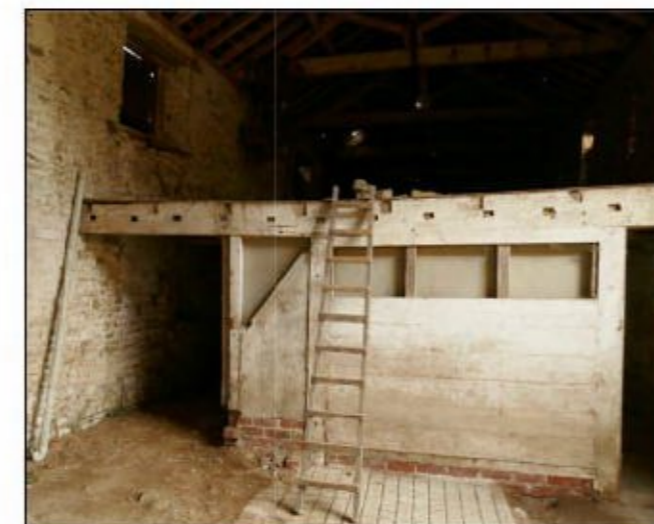
32 Remove section of existing floor to install new staircase to access loft.
