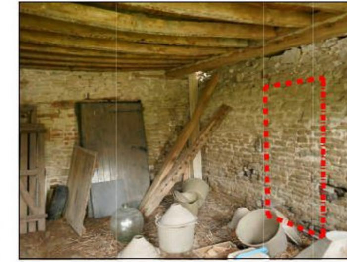
04 Create new opening for circulation at GF between proposed gym & recreational area.
