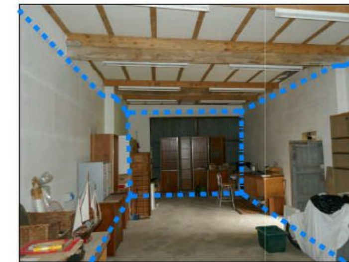
10 11 Remove modern internal lining to rediscover existing openings to North & South elevations.
