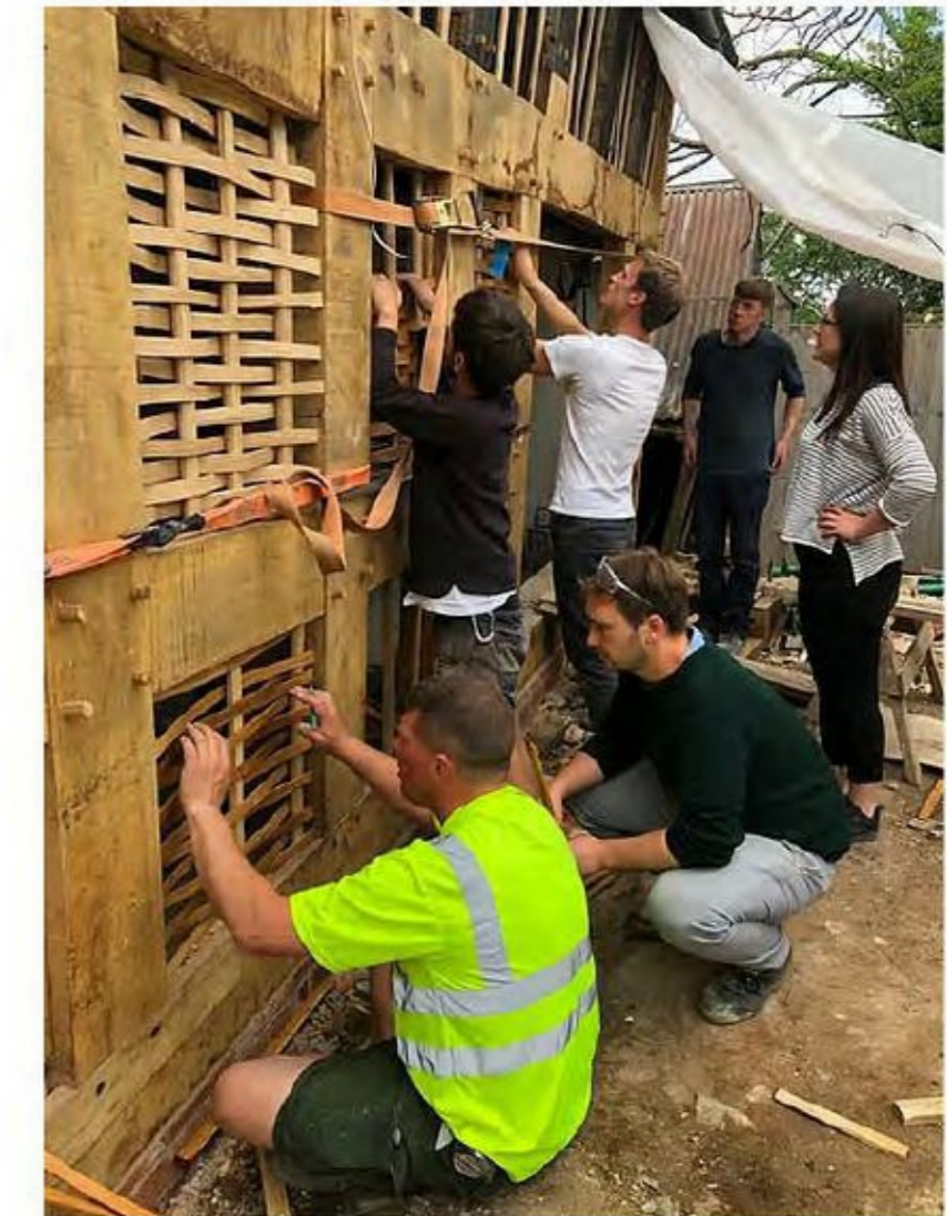
S.P.A.B. Scholars and fellows helping Paul Walters with the installation of wattle and daub panels
