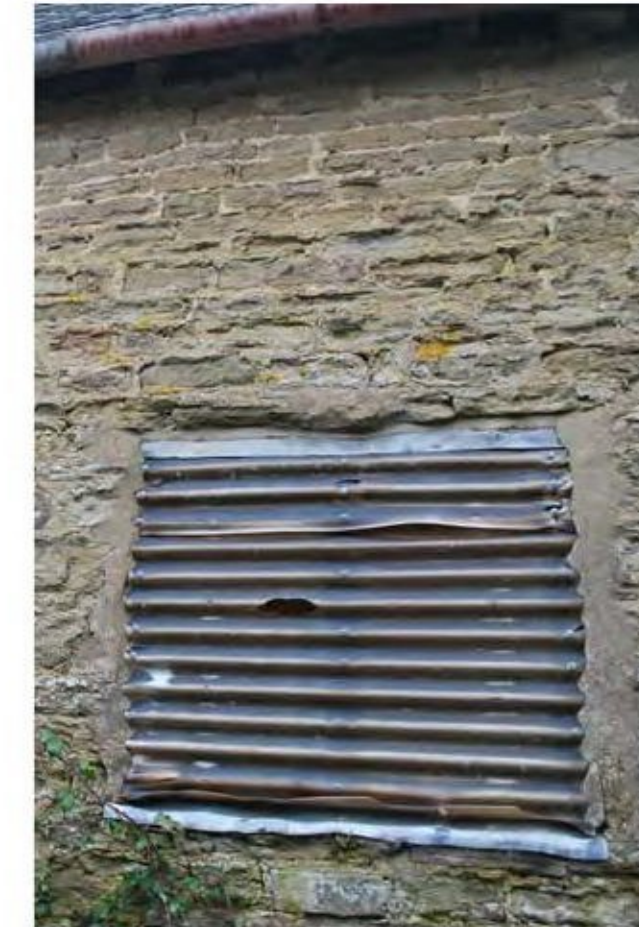
Photo 5. BARN 'B' - SOUTH ELEVATION BLOCKED LOFT ACCESS
