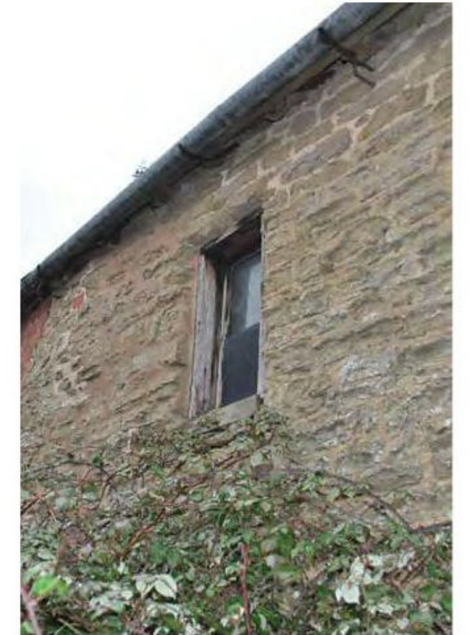
Photo 6. BARN 'B' - SOUTH ELEVATION BLOCKED LOFT ACCESS
