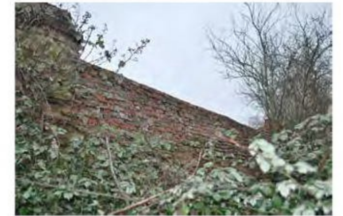
Photo 5B. GARDEN WALL TO WEST END PARTIALLY COLLAPSED (OTHER PROPERTY)
