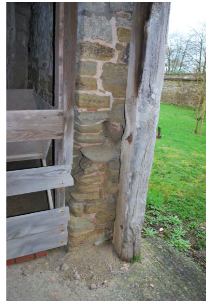
Photo 2. BARN 'A' - SOUTH ELEVATION DELAMINATED STONE
