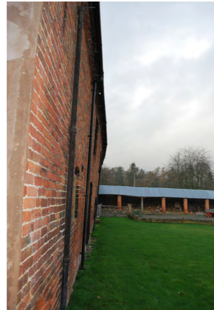
Photo 3. EAST WALL DISTORTION
