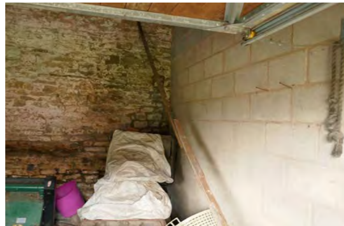
5. MODERN CONCRETE BLOCKWORK TO COACH HOUSE TO BE REPLACED
