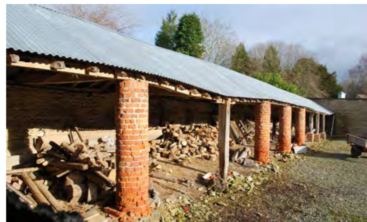
6. BRICK PIERS: MISSING PIERS TO BE REBUILT
