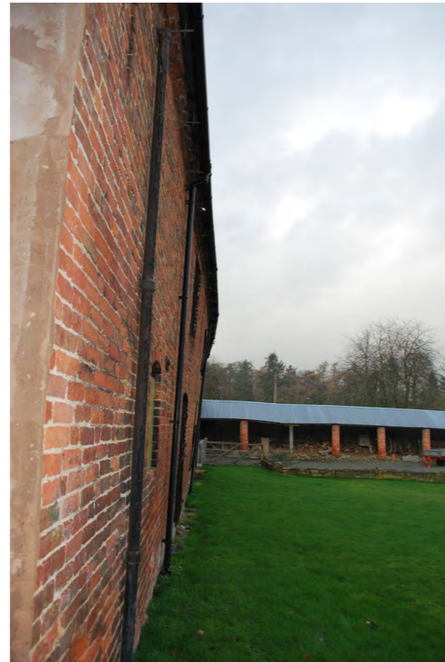
3. OUTWARD LEANING SOUTH WALL
