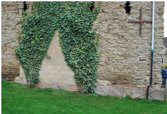
3. MODERN CONCRETE BLOCKS TO BE REPLACED
