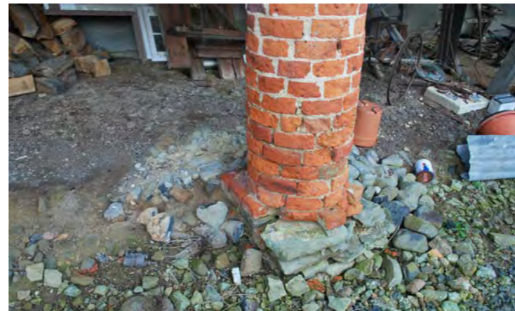
5. BRICK PIER BASES DAMAGED BY RISING DAMP
