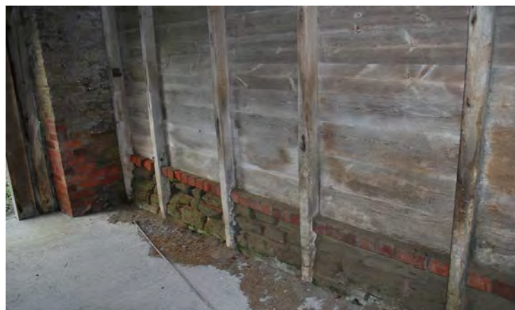
3. MODERN CONCRETE FLOOR AND DAMP IN DWARF RETAINING WALL
