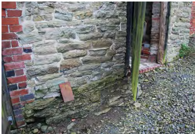
2. BRICK AND STONEWORK TO BE REPOINTED
