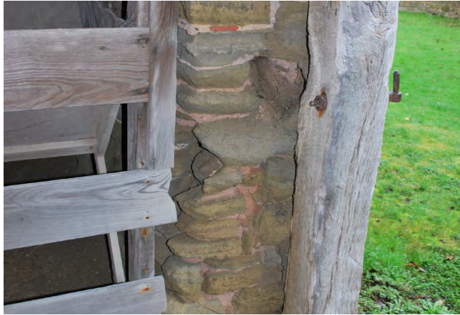
1. STONE PIER TO BE REBUILT
