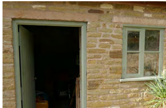
6. MODERN BLOCKWORK & STONE ELEVATION WITH CONCRETE LINTELS TO BE REPLACED
