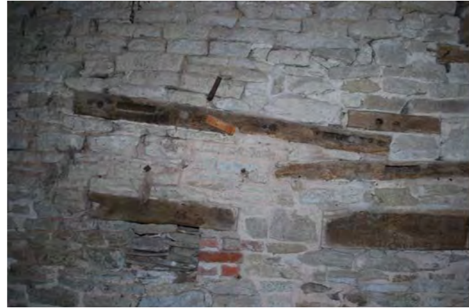
4. STRUCTURALLY FAILING STONE WALL NEEDING TO BE TIED TOGETHER
