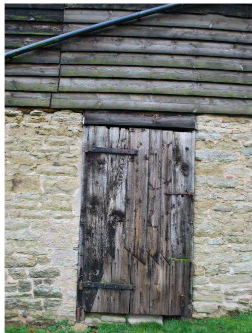
3. HISTORIC DOOR WITH SPAB REPAIRS
