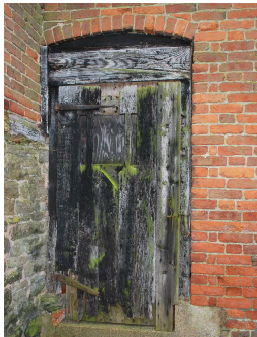
2. HISTORIC DOOR VERY BADLY ALTERED
