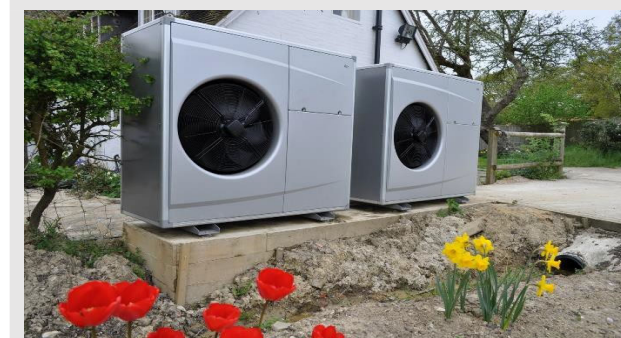
Outdoor units of an ASHP system (discharge)
