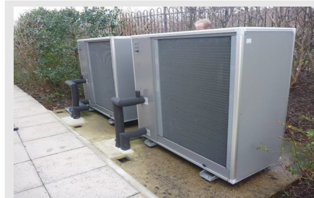
Outdoor units of an ASHP system (intake).
