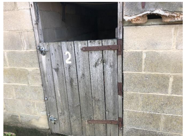
Photo 16: Door on western side of B11, with small gaps around door frame
