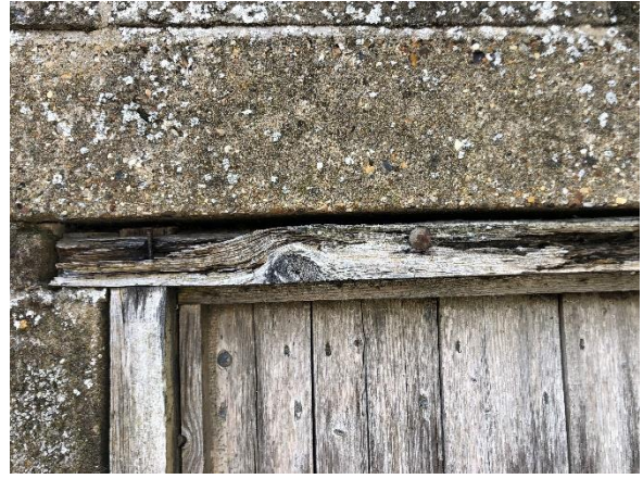
Photo 18: Gap above door frame of B12
