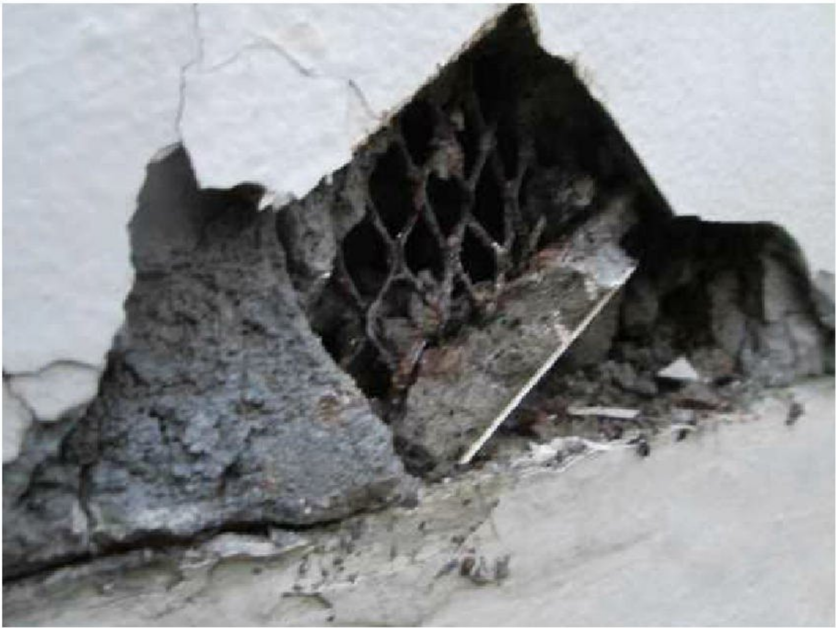
Corroded Galvanised Mesh
