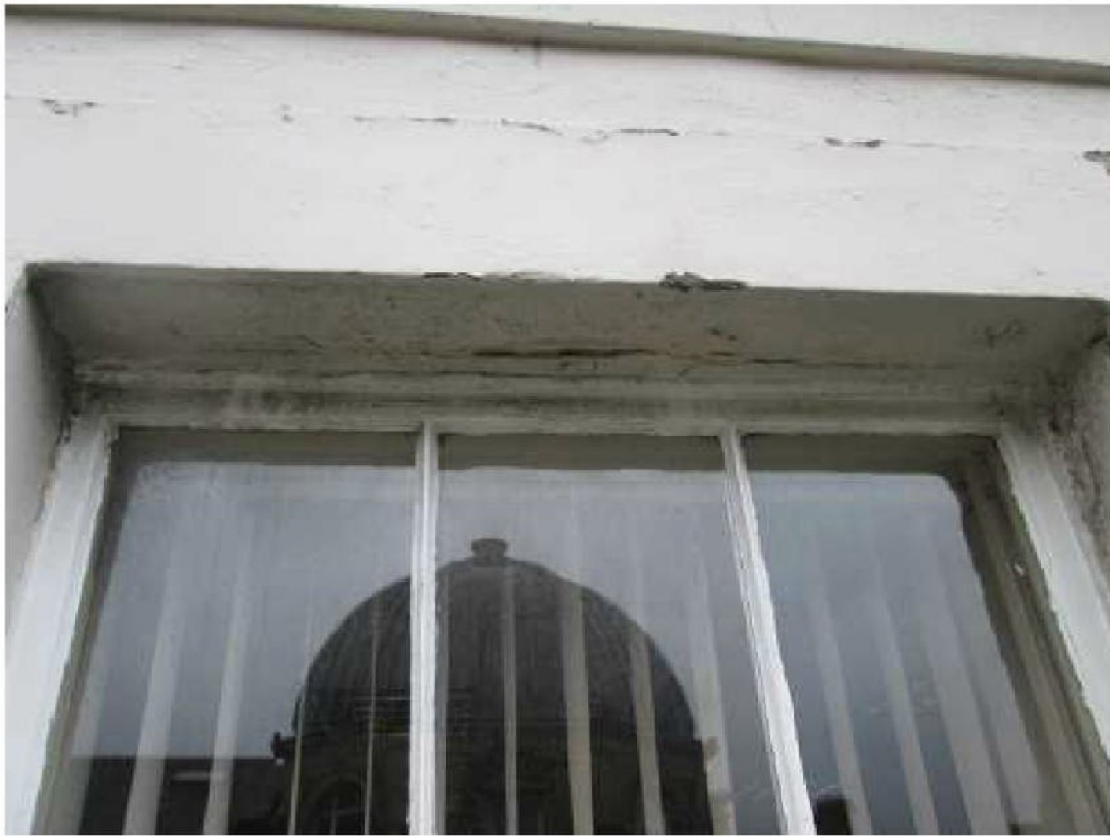
Window "Painted Shut"
