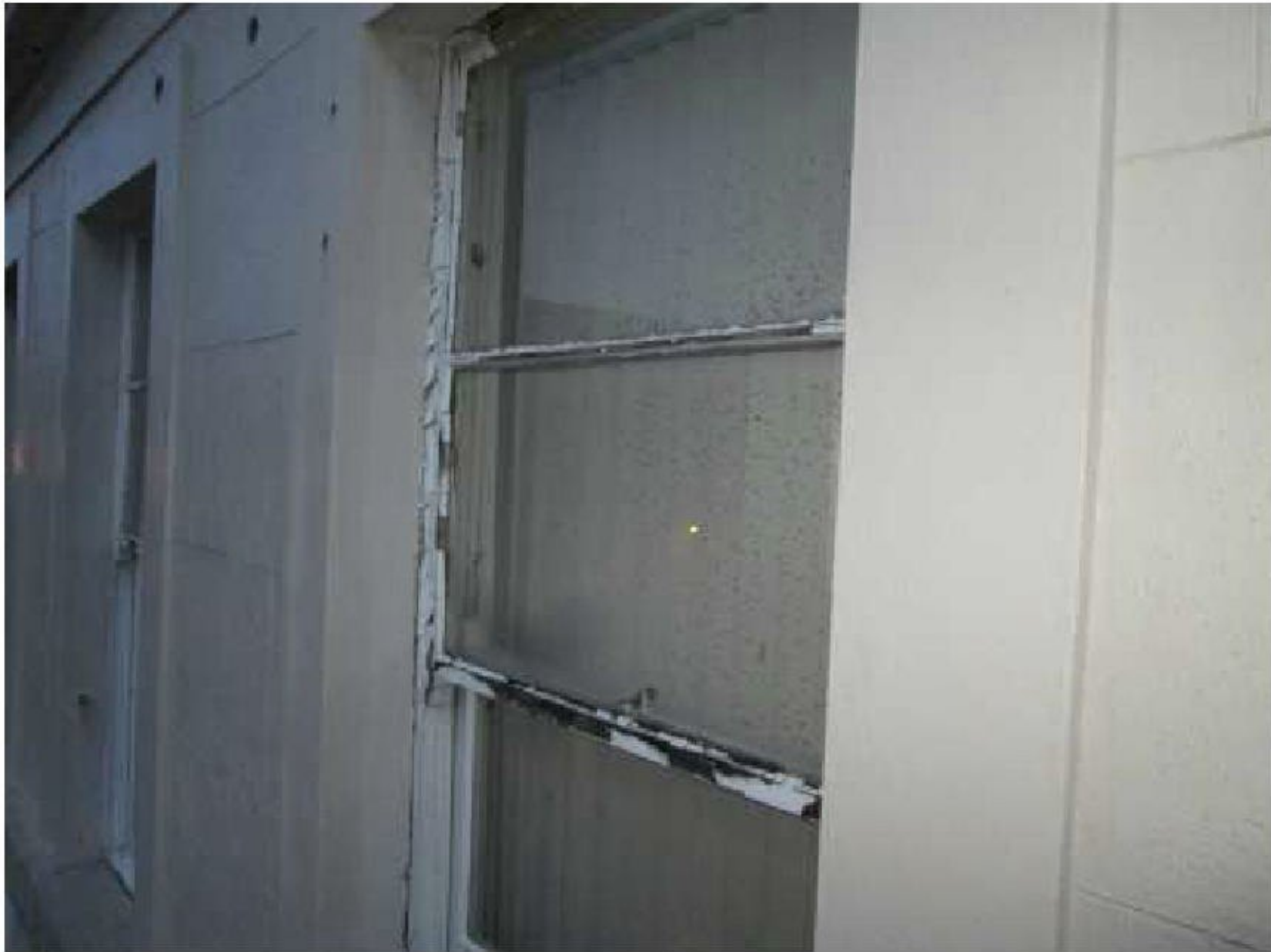
Poor Decoration and Defective Putty
