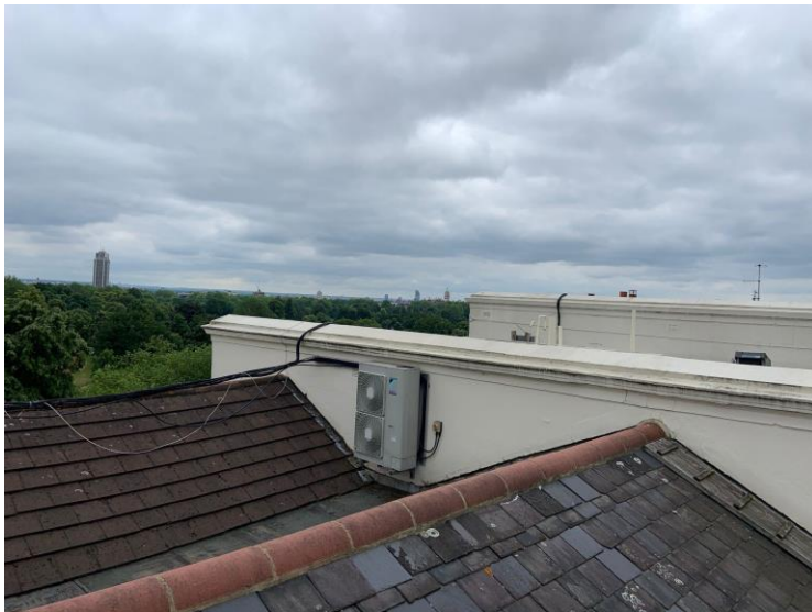
Number 26 – flat 4/5 - Example Air condenser Showing air condenser unit at roof level.
