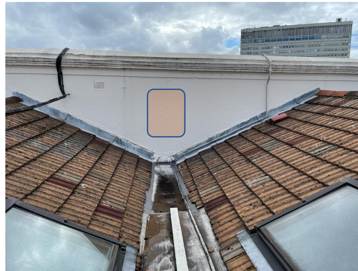
Flat 9 – Roof level highlighting the area for the proposed air con unit.
