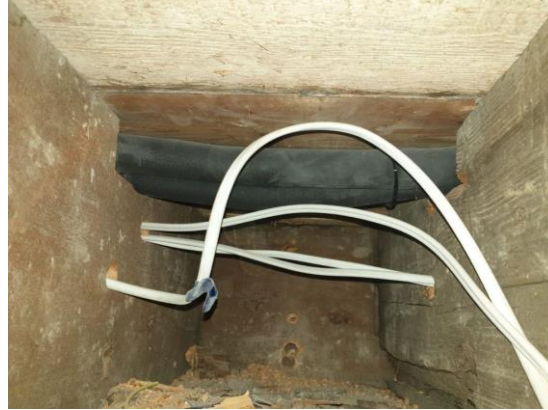
2 nd Floor; Existing cables under boards
