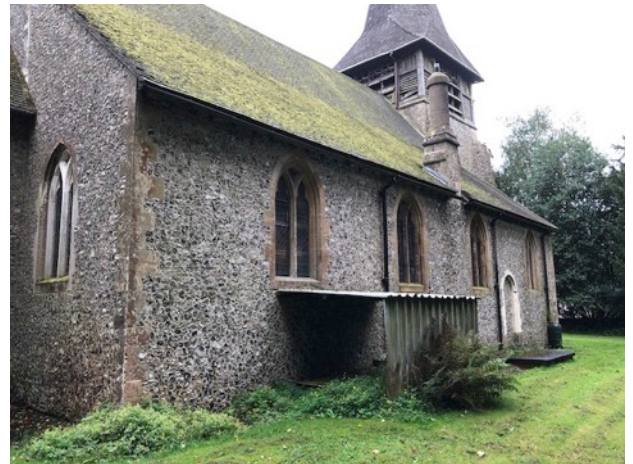
4 North Aisle viewed from the east. The enclosure in the foreground is above the oil tank
