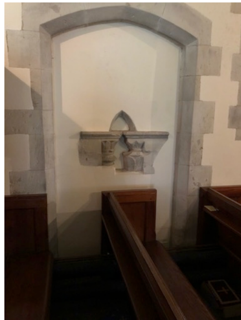
5 Blocked-in doorway in the North Aisle. Fragments of Norman masonry have been embedded in the wall
