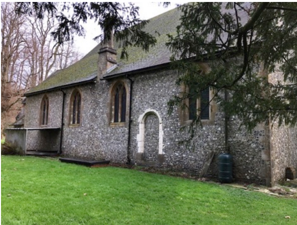
3 North side of the North Aisle. It is planned to utilise the old doorway for access to the extension.
