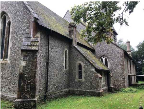
5 General view of north side of the church, viewed from the east: Chancel and Vestry in foreground.
