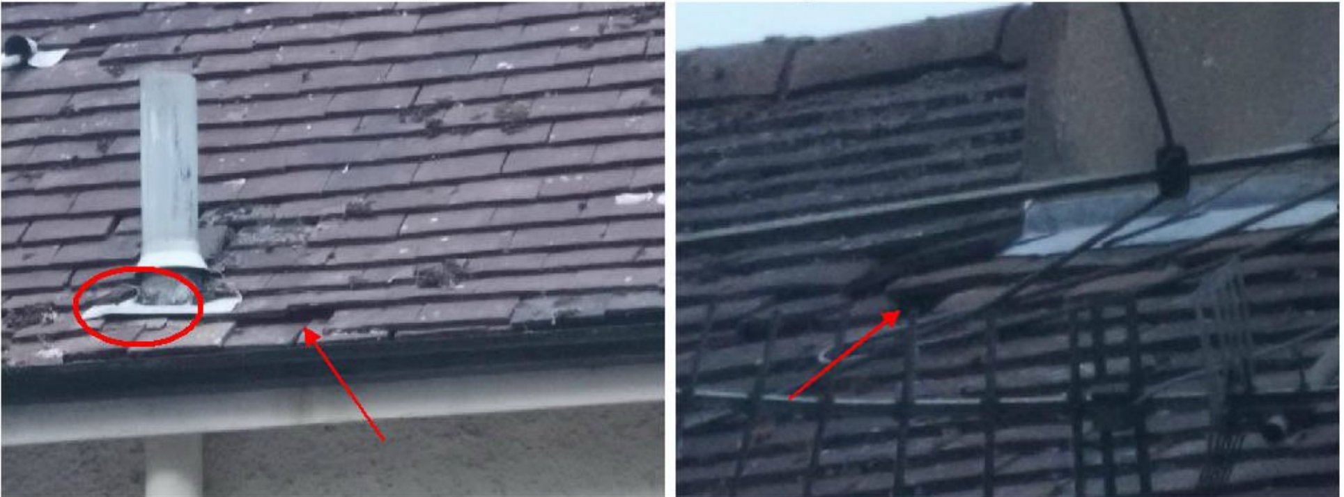
Figure 3. Example of gap under lead flashing/roof tile and missing tile
