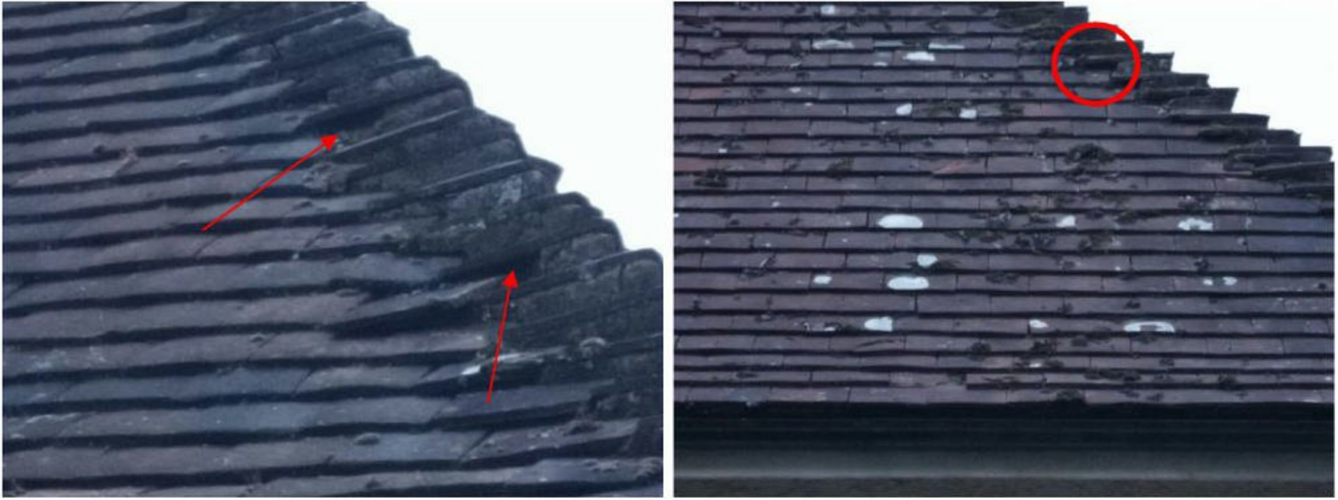
Figure 4. Example of missing mortar below bonnet tiles
