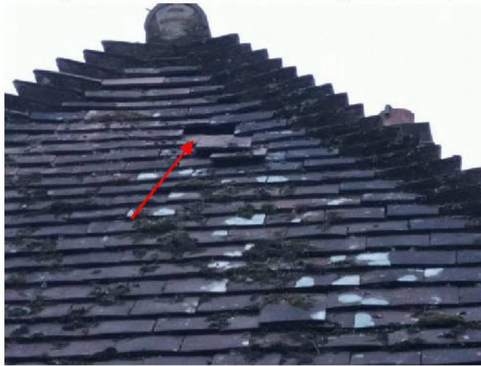
Figure 2. Example of missing roof tiles
