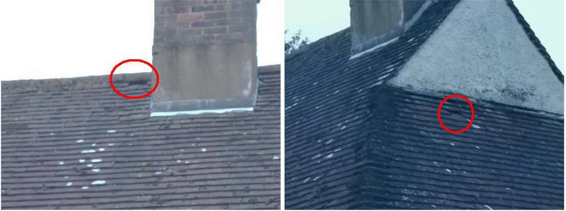
Figure 1. Example of missing roof tiles
