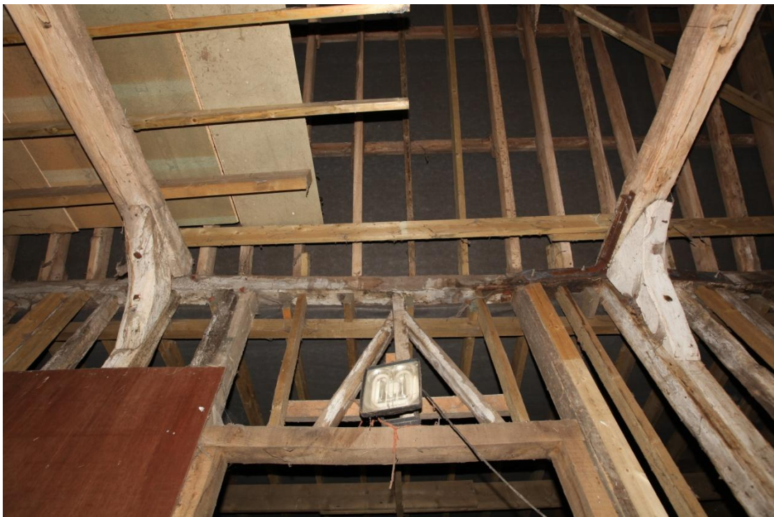
Illus. 12. A detail of the rear (southern) roof-plate of the central bay showing its original central stud and primary braces with replaced studs on both sides. The knee-braced tie-beams are original to the structure but re-used as they contain pegged mortices for arch-braces while the posts lack both jowls and arch-brace mortices.
