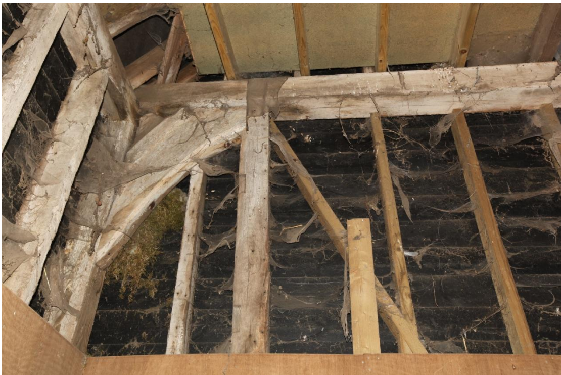
Illus. 16. The original bolted knee-brace in the barn's north-eastern corner with no stud mortices in the tie-beam, proving that either a fourth bay has been lost or the present three-bay structure was designed as an extension to a pre-existing building on the east. The unpainted studs to the right date only from 2003.
