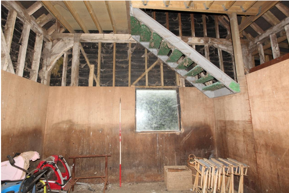
Illus. 15. The eastern internal gable showing the original knee-braces of an open truss with inserted studs beneath the tie-beam. Most of these studs consist of modern softwood but some appear older and in situ so the truncation occurred before the barn was refurbished in 2003 – as confirmed by the 1984 listing description which refers to the present three bays.
