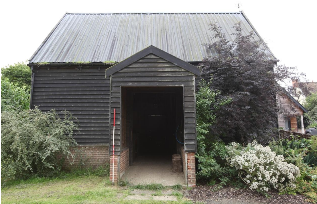
Illus. 5. The northern exterior of Barn 3 showing the newly added porch of 2003 and the replaced corrugated iron roof of the same date.
