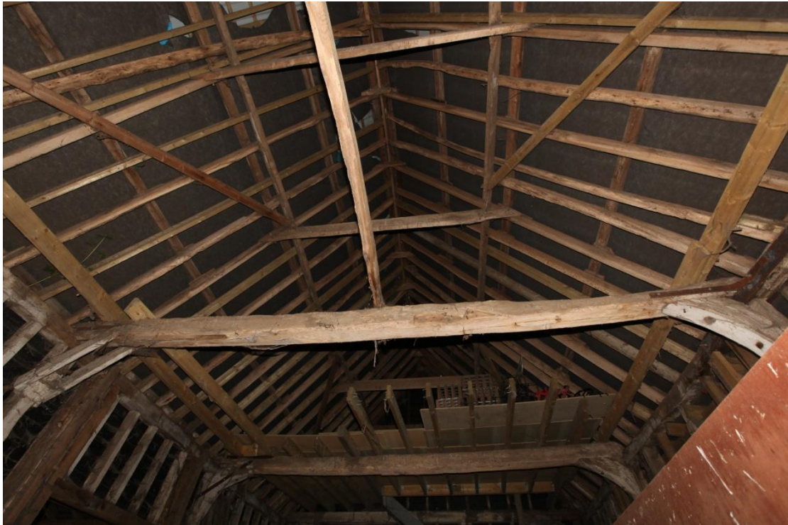
Illus. 11. The roof structure from the west showing the empty arch-brace mortices in the re-used western tie-beam with the same features in the eastern tie beam beyond. The collars of the clasped-purlin structure are both pegged and nailed in an apparently original arrangement and the purlins are narrow-sectioned. Some rafters were re-used when new while others are modern replacements but the ridge-board is original.
