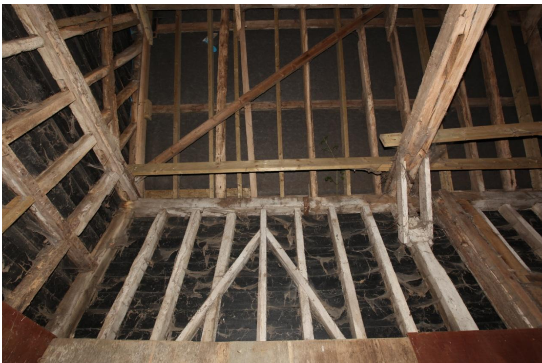
Illus. 14. A detail of the original framing of the western bay's northern interior showing its narrow-sectioned timbers and nailed braces along with the twin plank-sectioned braces that replaced an original knee-brace to the wall post on the right.
