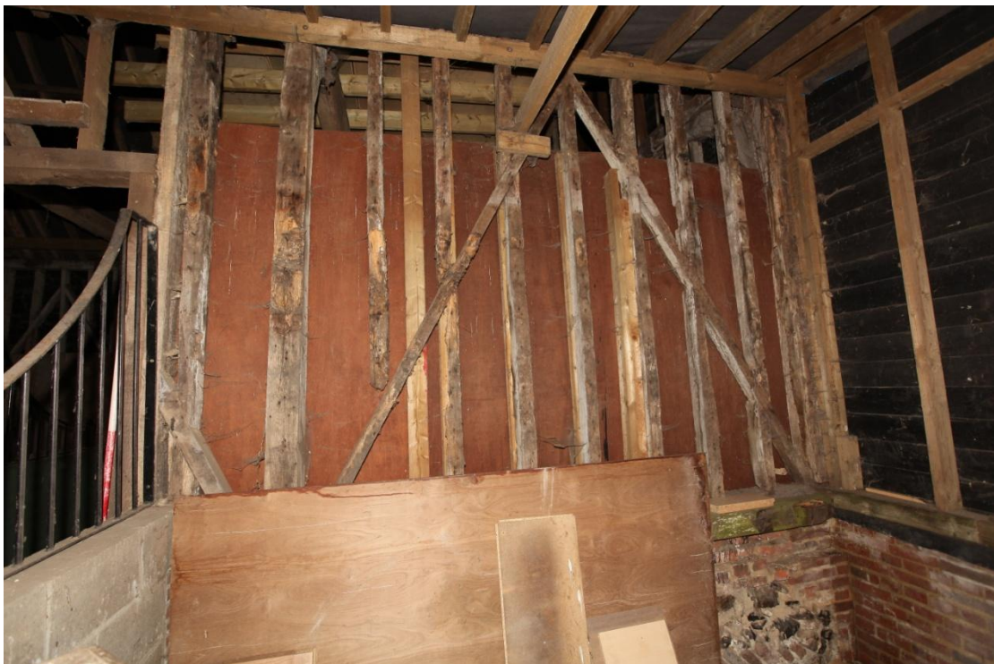
Illus. 18. The southern exterior of the main barn's eastern bay from the modern lean-to extension showing its intact framing and flint-rubble plinth. This feature is mentioned in the listing description but the plinth has since been largely rebuilt in brick. Combinations of flint and diagonal brickwork of this kind are typical of Victorian rather than Georgian work.
