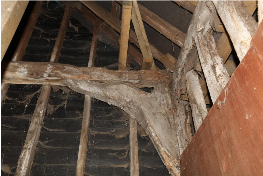
Illus. 17. The original bolted knee-brace in the barn's south-eastern corner with no mortices in the tie-beam. With its counterpart on the north (illus. 16) this demonstrates that the structure lacked a solid wall on the east and either continued or was designed as an extension to an older building.
