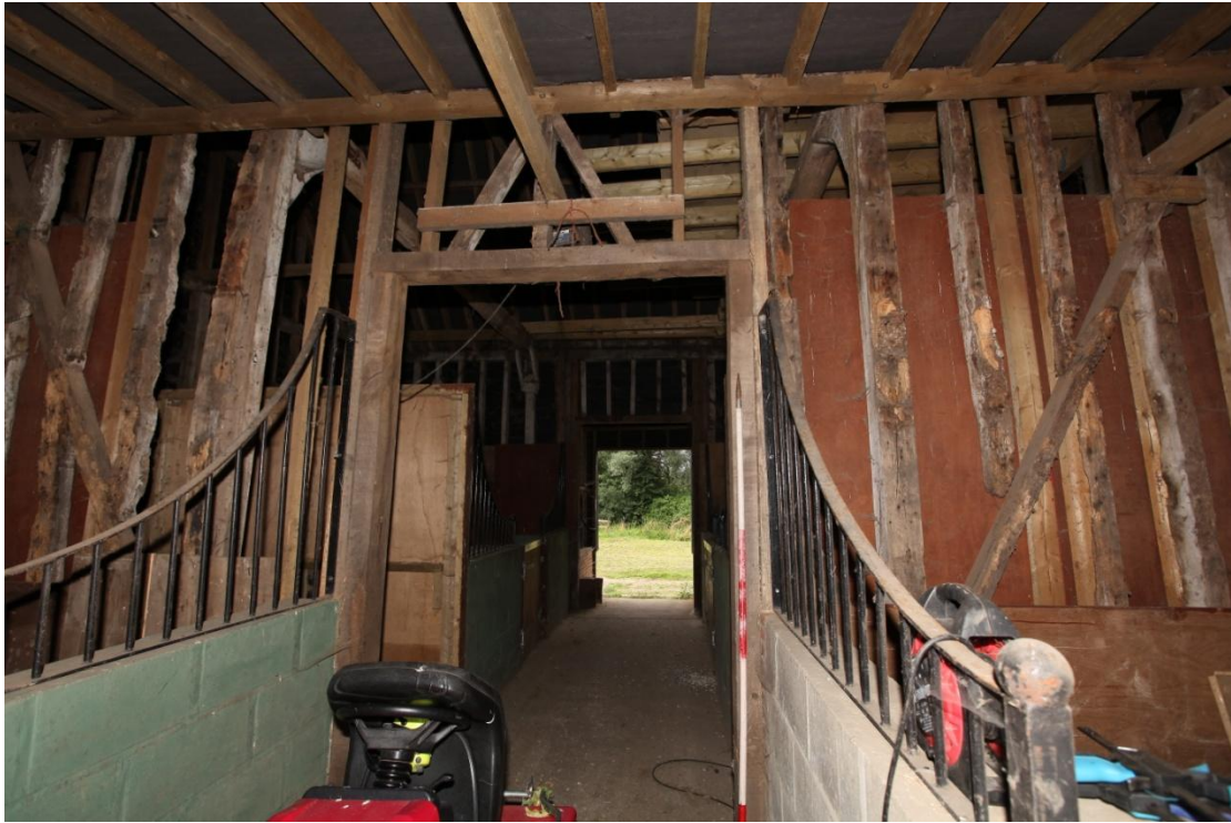
Illus. 19. The southern exterior of the central bay from the lean-to showing the modern door frame cutting the original central stud and braces with the intact studs and diagonal primary bracing of the outer bays on each side.
