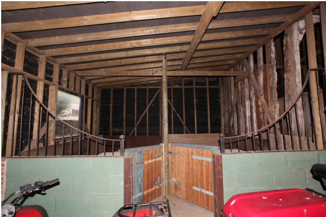
Illus. 20. The southern lean-to of 2003 from the east showing its recent softwood fabric and loose boxes with the exposed framing of the main barn to the right. This lean-to replaced but replicated the open-sided lean-to shelter or cart lodge shown on the Ordnance Survey of 1958 and the aerial image of circa 1970 (figures 7 and 9).
