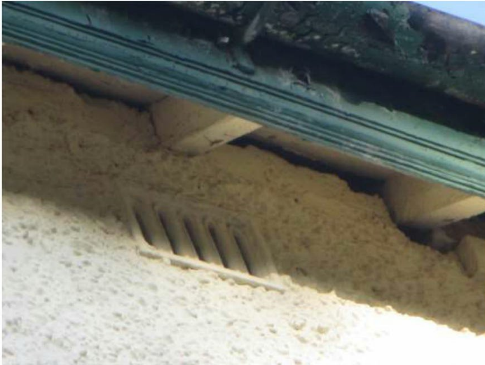
Photograph 7 – Gaps at the eaves and around the protruding rafters on the eastern aspect of the building.
