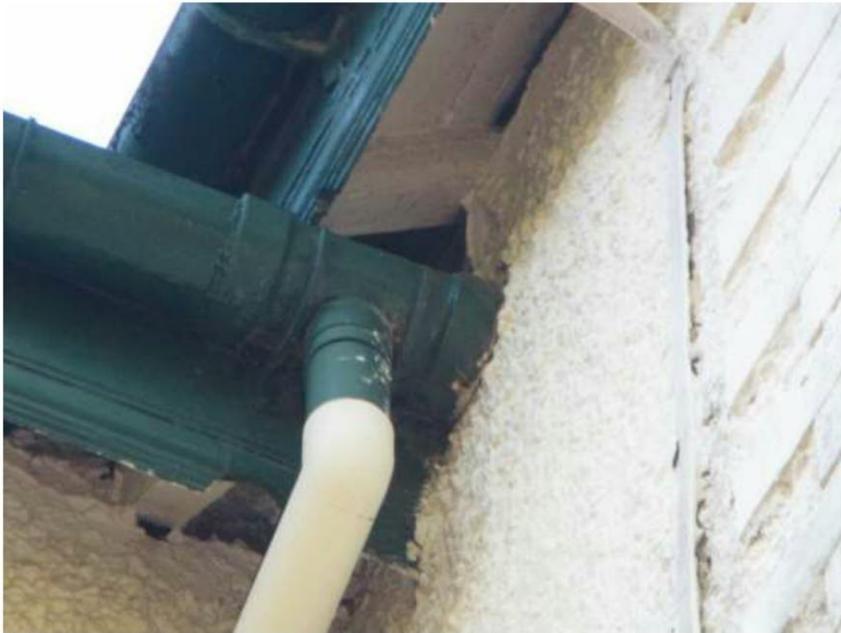
Photograph 6 – Gaps at the eaves on the western aspect of the building.
