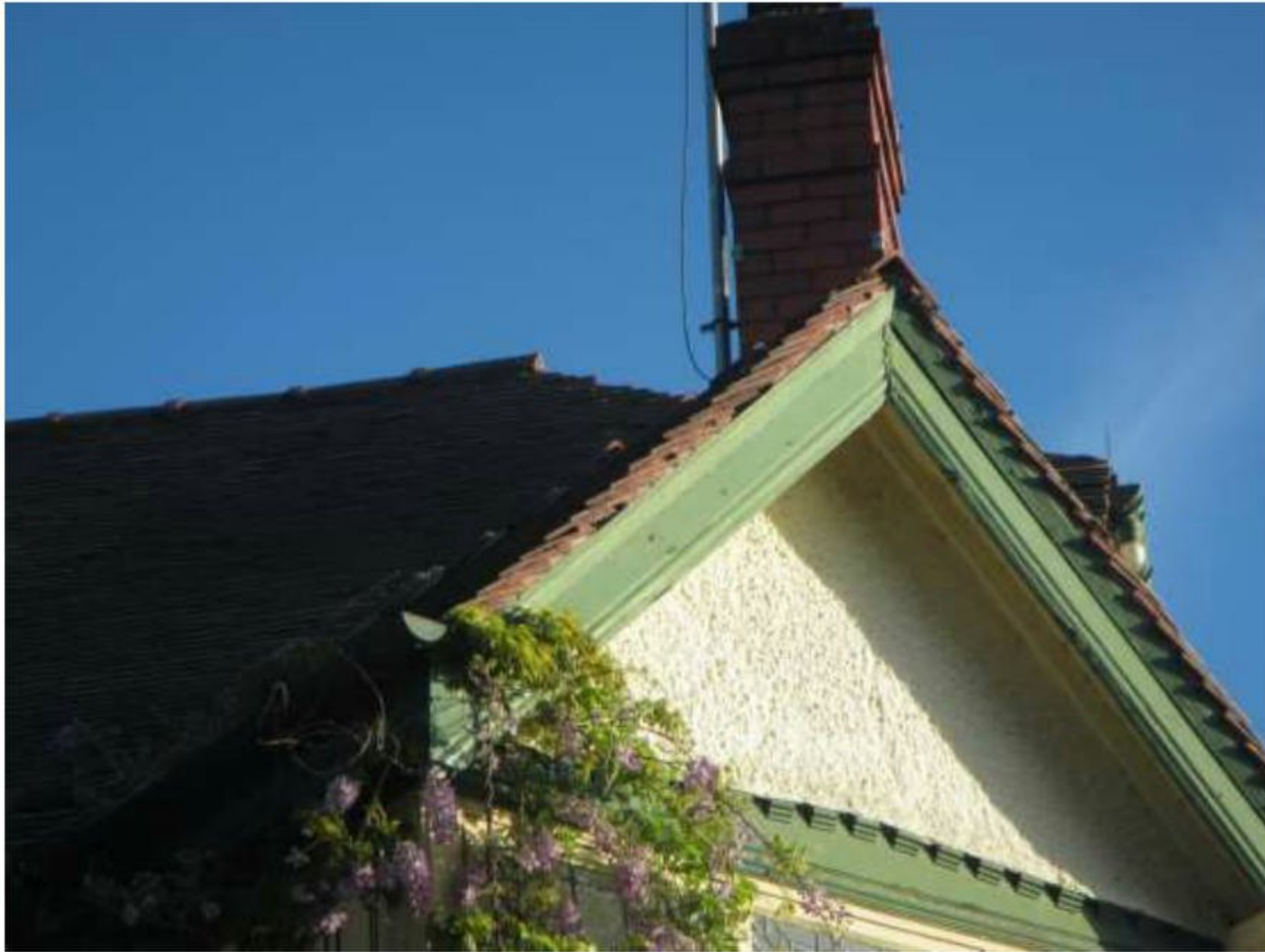
Photograph 3 – Example of gaps where mortar is missing from the end roof tiles.
