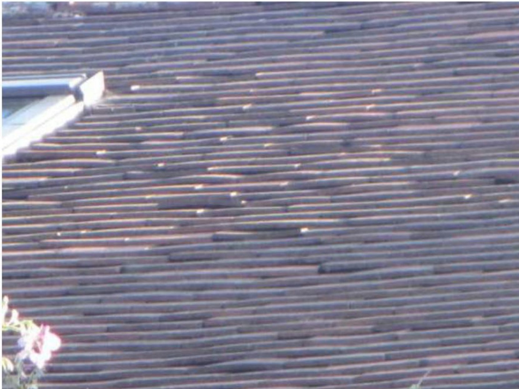
Photograph 2 – Numerous lifted roof tiles on the southern aspect of Building 1.
