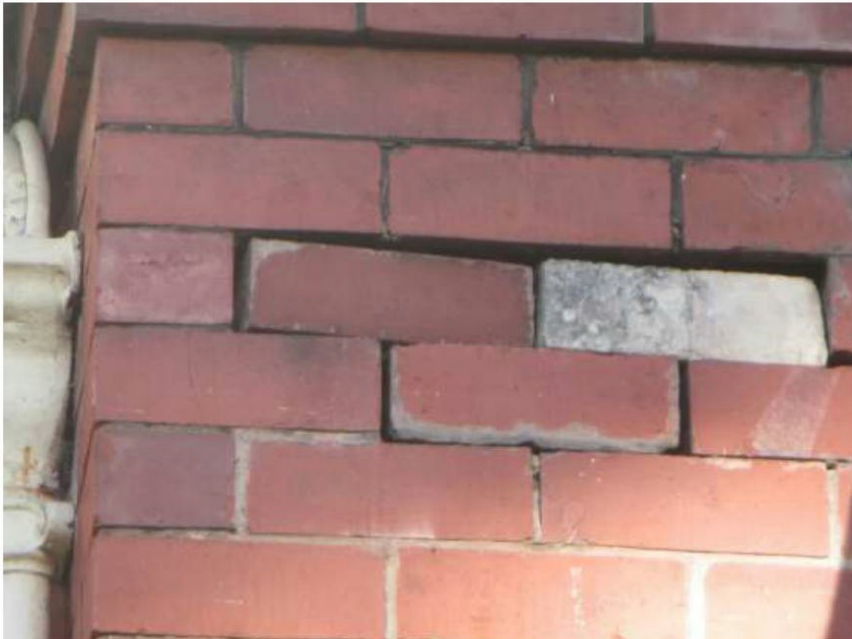
Photograph 10 – Gaps in the brickwork on the eastern aspect of the building.
