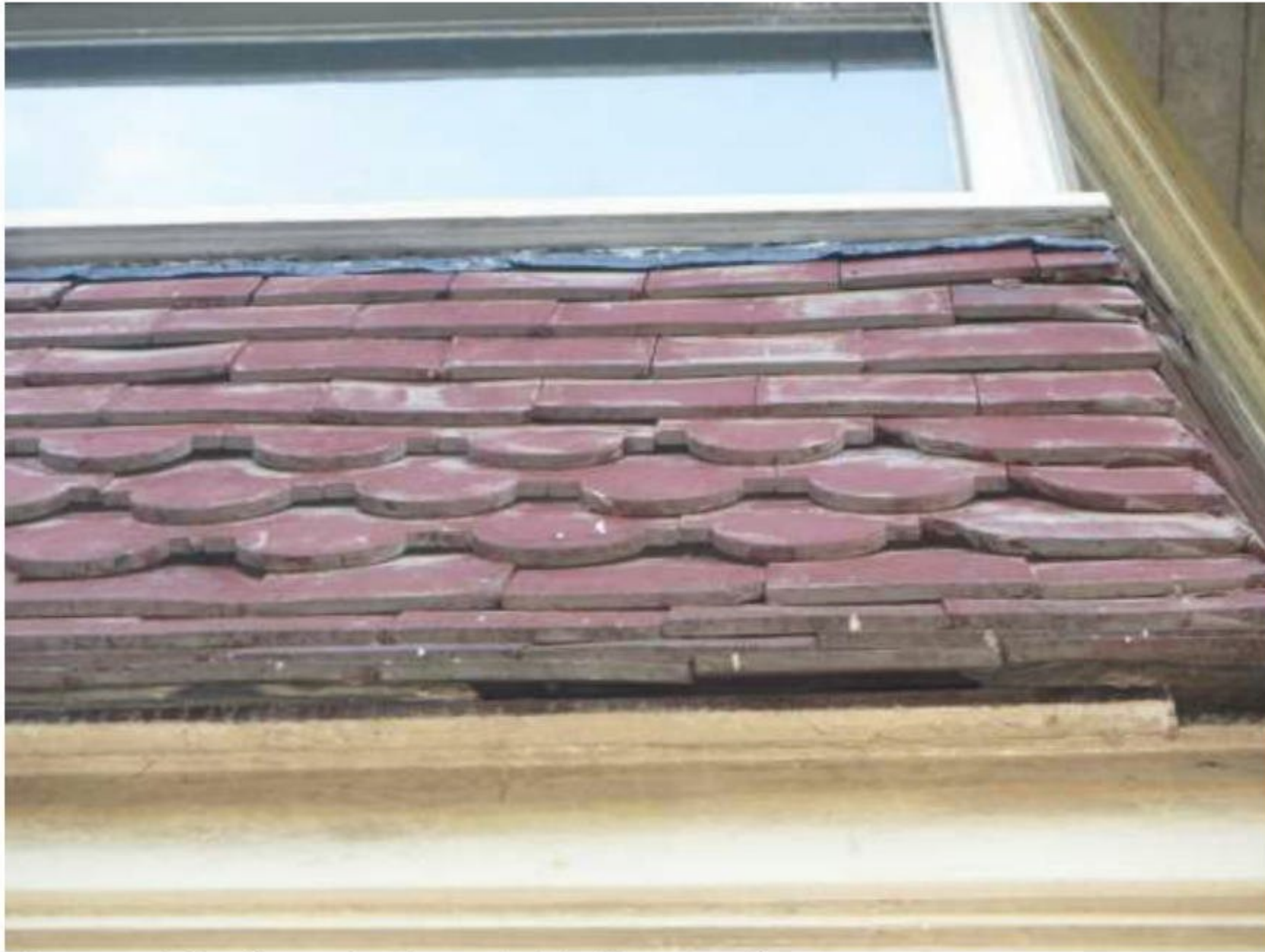
Photograph 9 – Example of gaps behind hanging tiles.
