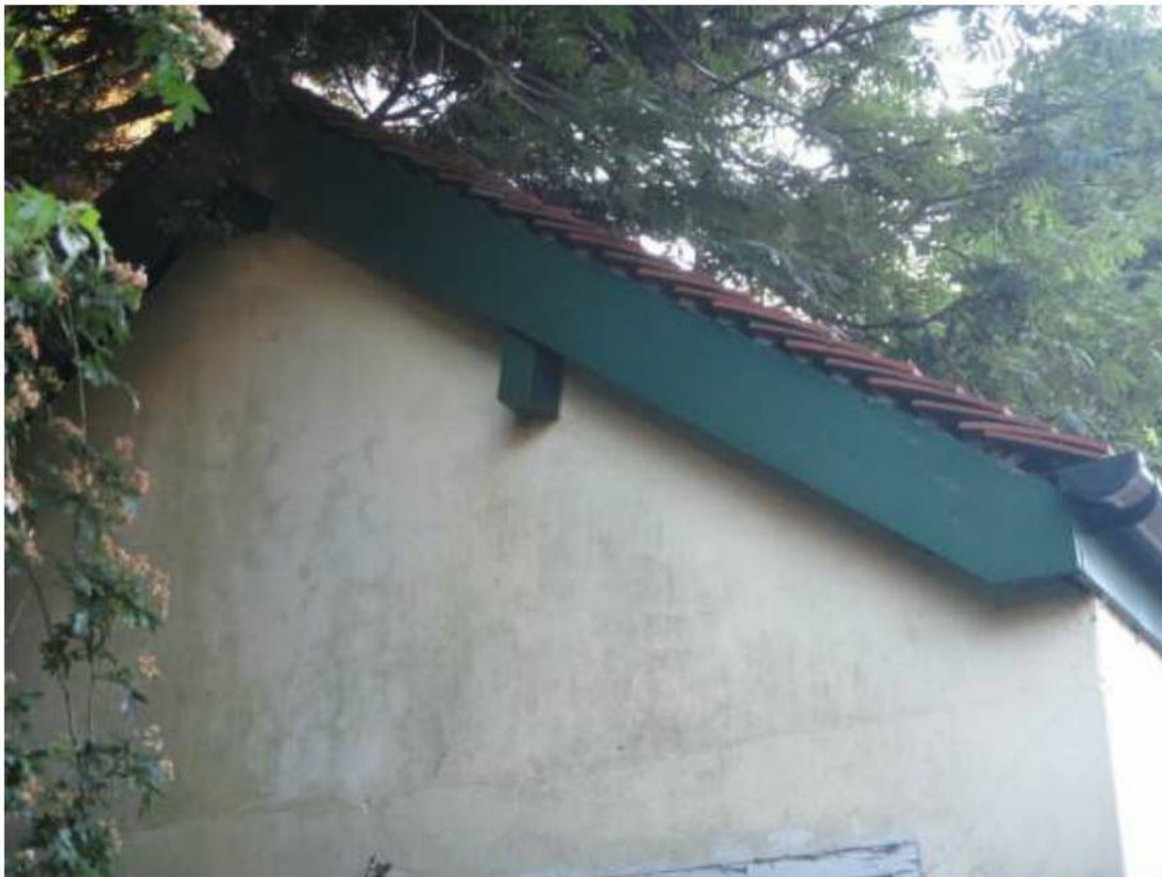
Photograph 14 - View of gaps at end roof tiles of garage.
