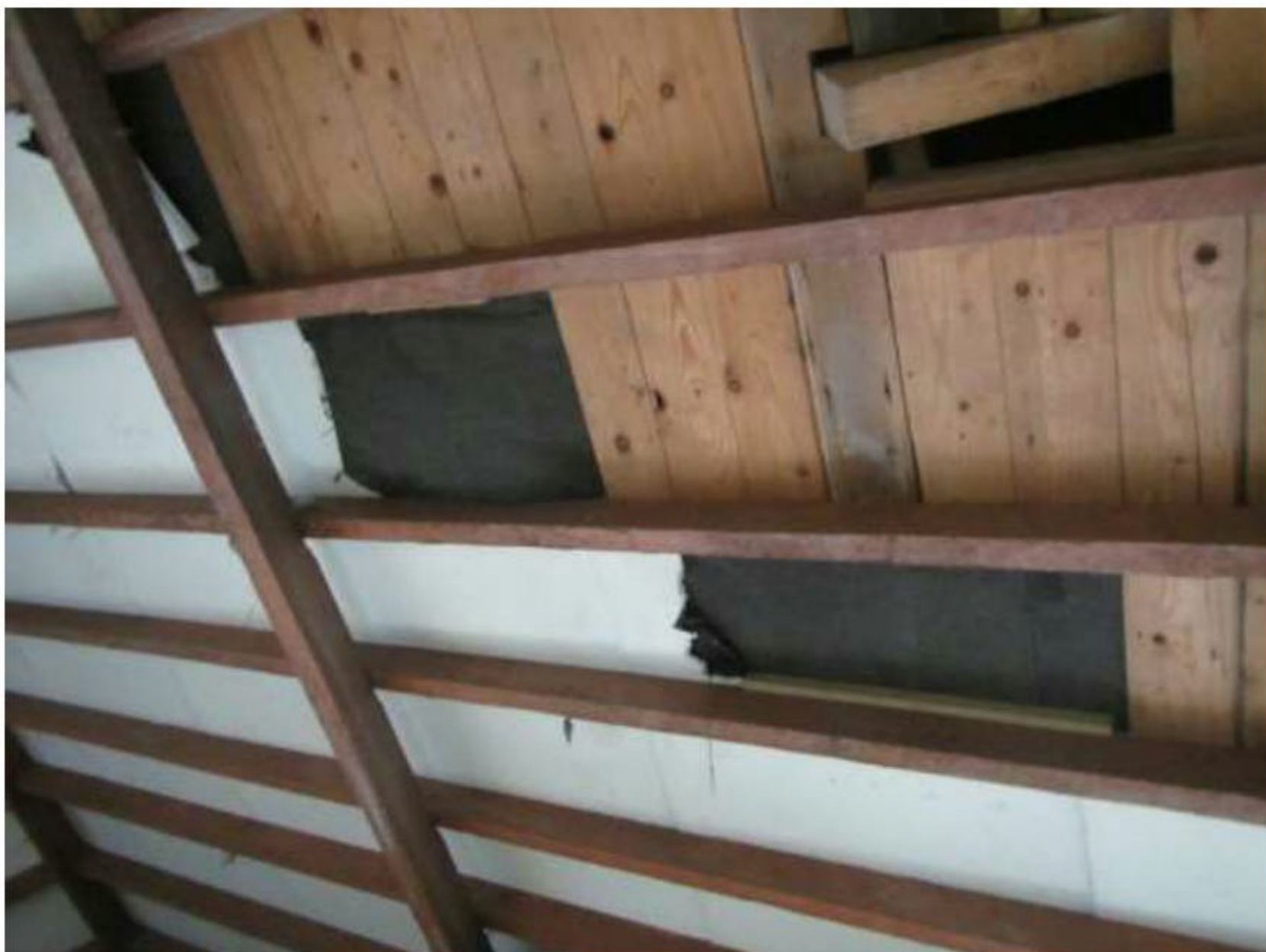
Photograph 20 – View of roof linings; polystyrene sheets, bitumen roofing felt and wooden sarking boards.
