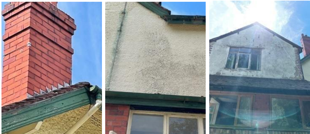
Weathered stacks & poor external render coverings
