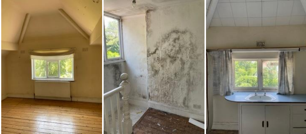
External walls affected by damp penetration
