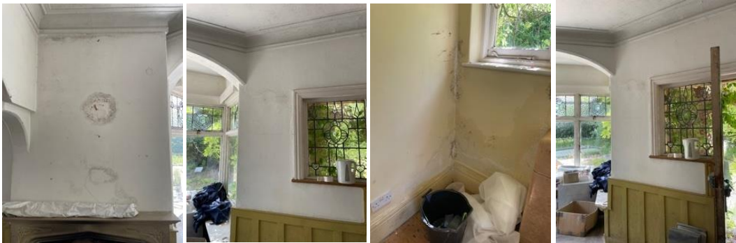
Damp affected wall plaster
