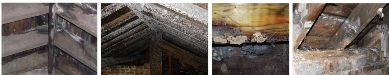
Wet rot in roof timbers
