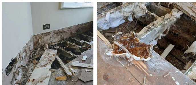
Dry rot in floor Joists
