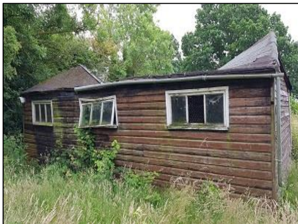
Figure 1: The billiards hall with collapsed roof.
