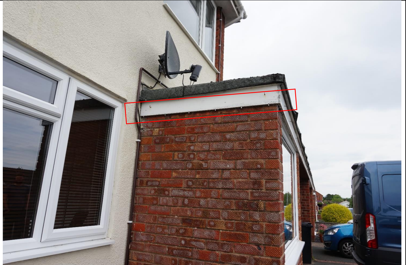
Figure 4: Gap on western edge of porch
