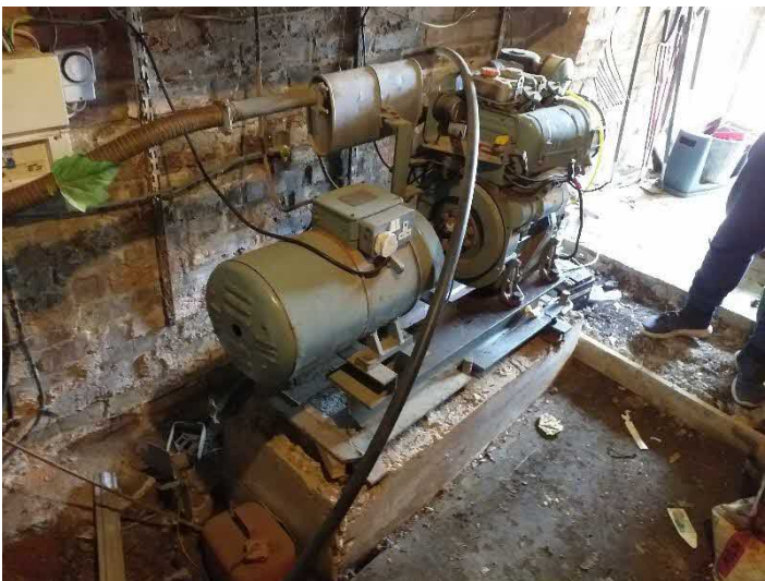
Photo 11: View of generator which will require removal to allow access to the soils below.
