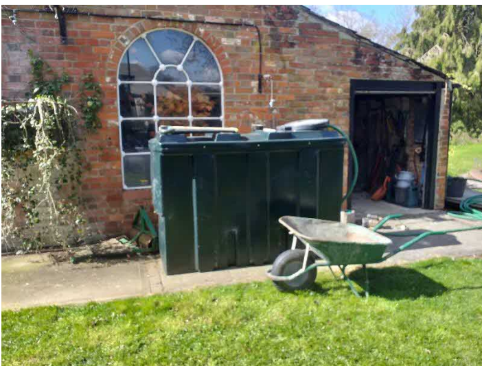
Photo 3: Temporary OST installed to maintain a supply of fuel to the boiler. Boiler located through garage door on the right.
