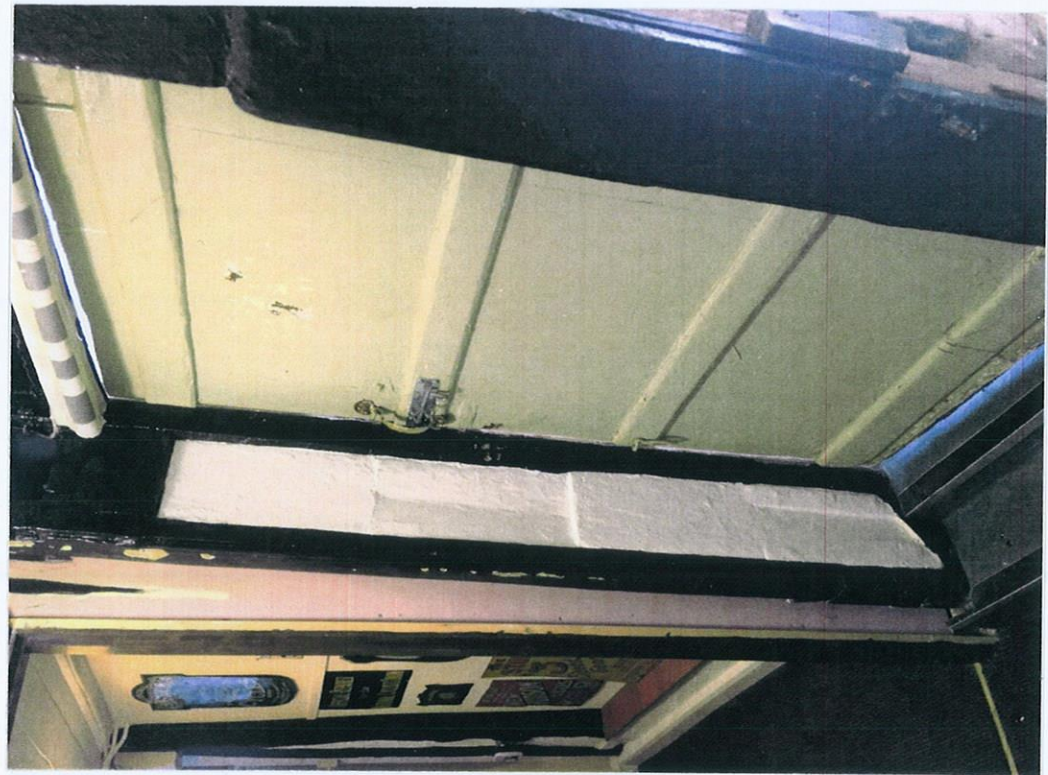
REMOVE EXISTING CORRIDOR PARTITION. DIVIDING PARTITION TO BE REMOVED AND CHANGE IN LEVEL TO BE PROVIDED WITH TEMPORARY HANDRAIL AND BALUSTRADE UNTIL FLOOR SLAB IS REDUCED TO 'CORRIDOR' LEVEL.
