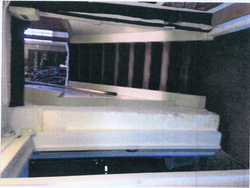
CORRIDOR VIEW. : SHOWER ROOM DOOR ON LEFT. : PARTITION ON RIGHT TO BE REMOVED. : HISTORIC DOOR AND FRAME TO BE RETAINED ON RAISED KERB.
