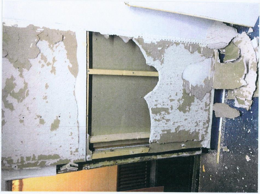
REMOVE EXISTING CORRIDOR PARTITION. DIVIDING STUD AND PLASTERBOARD PARTITION TO BE REMOVED AND CHANGE IN LEVEL TO BE PROVIDED WITH TEMPORARY HANDRAIL AND BALUSTRADE UNTIL FLOOR SLAB IS REDUCED TO 'CORRIDOR' LEVEL.
