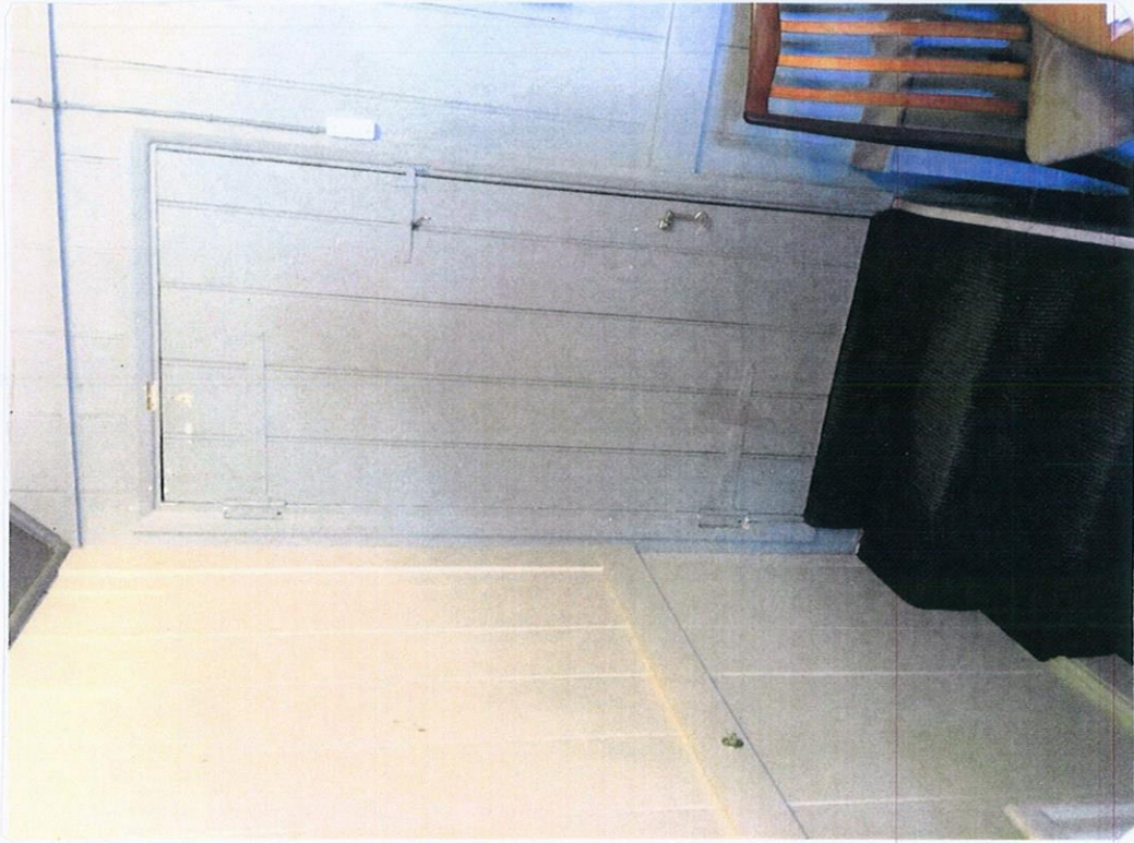
STEPS UP TO 'KITCHEN' STAIR UP TO PUB FLAT (KITCHEN). BOARDED DOOR AND WALLS. CARPETTED STEPS.
