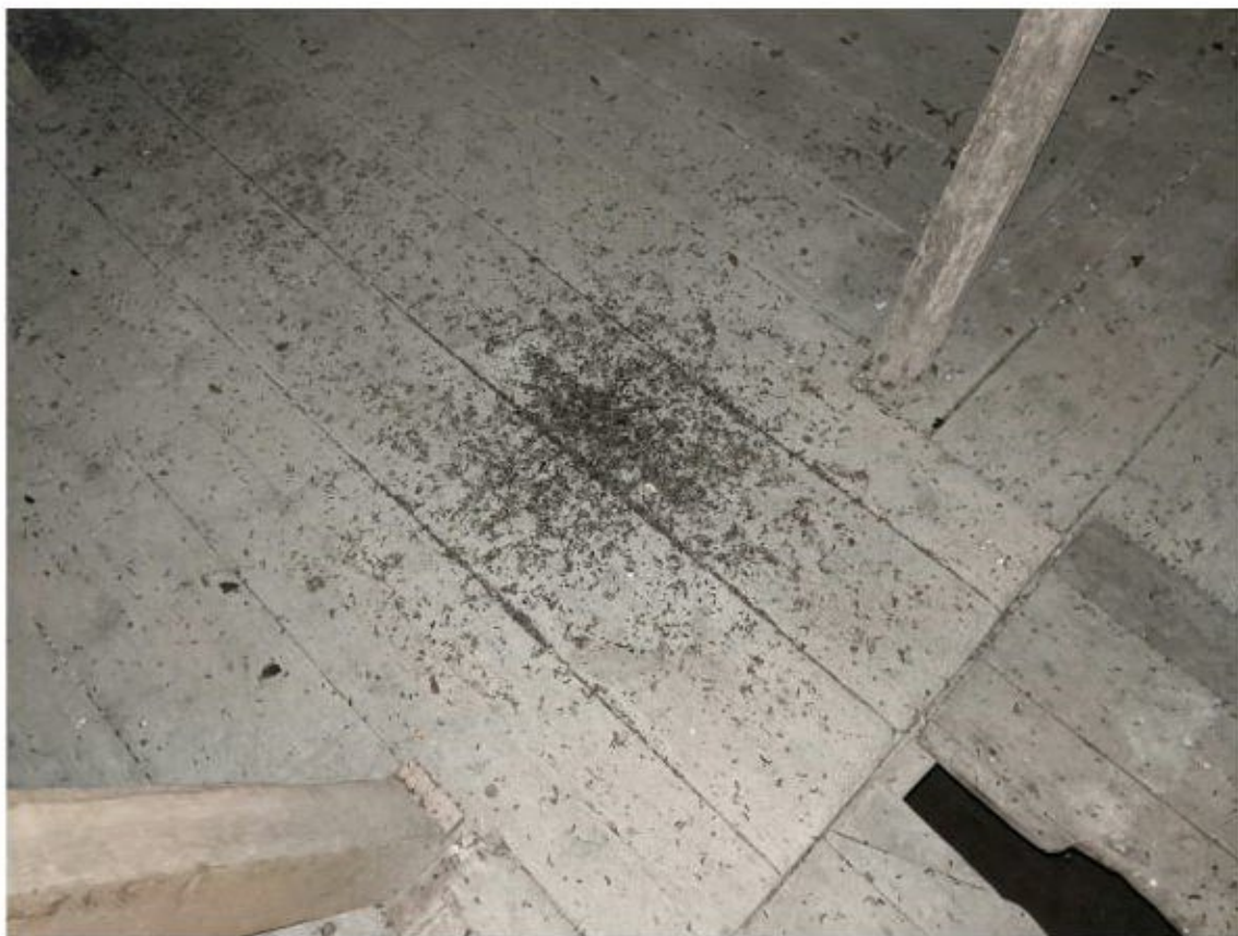
Photo 4 BLE dropping in loft space
