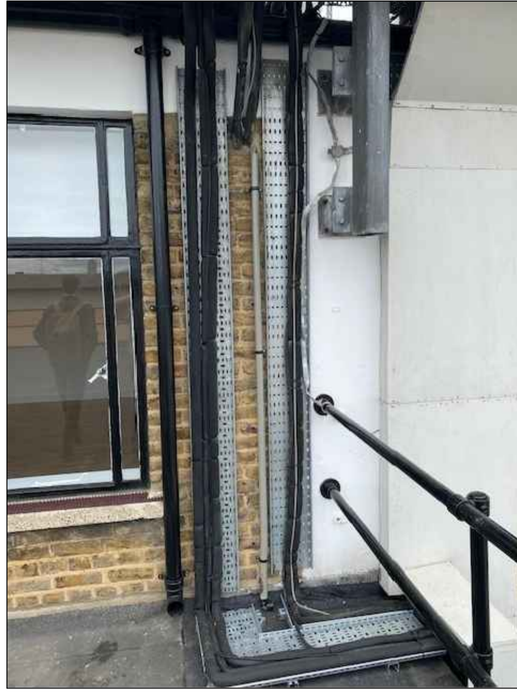
Image 1 Existing tray work to be used
