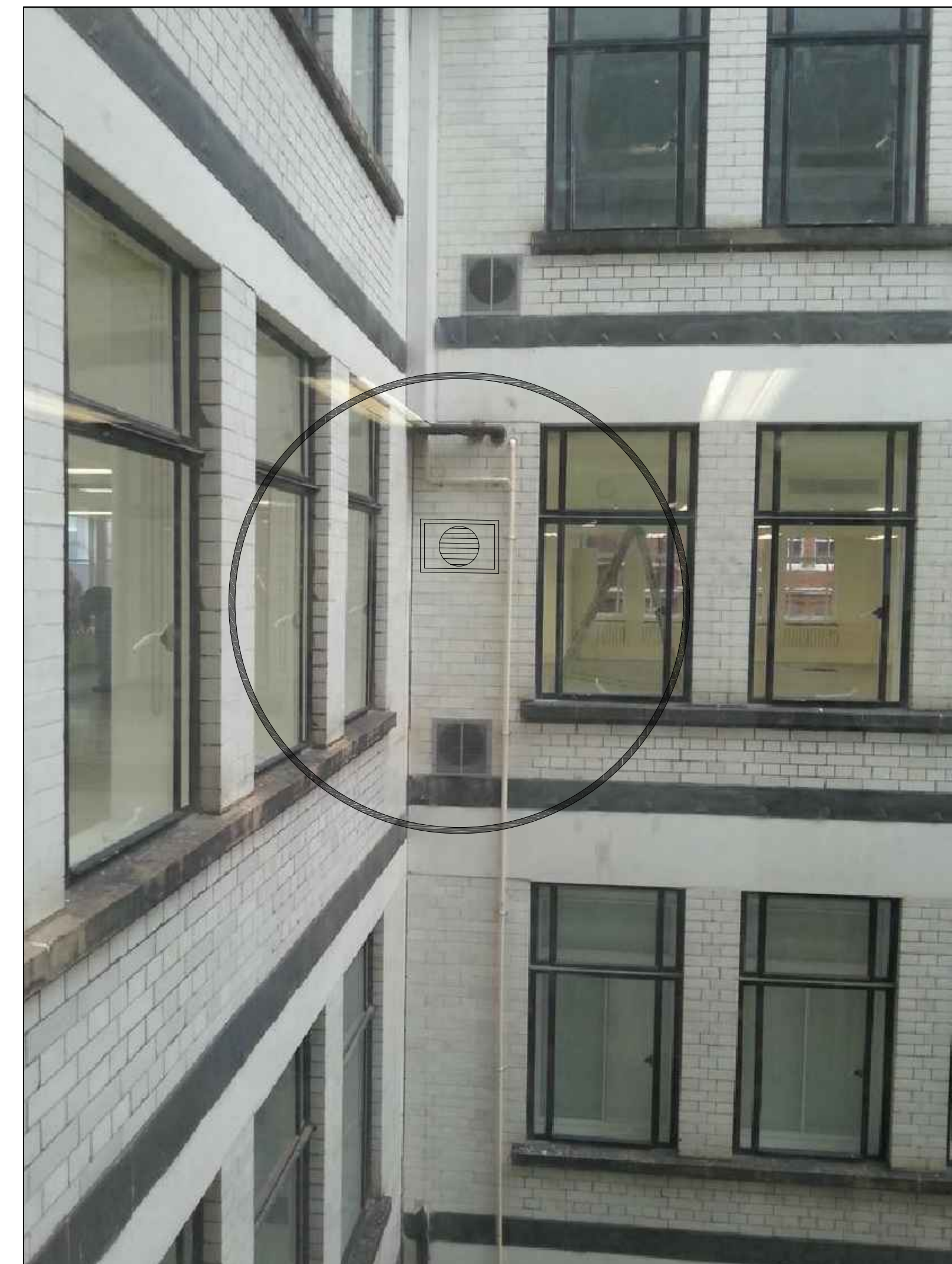
Typical External View
