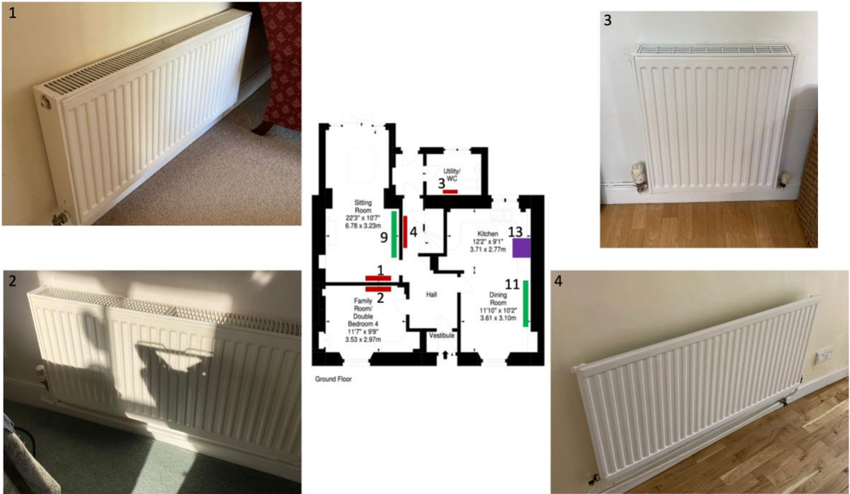
Figure 7: Photos of old radiators we propose to replace on the ground floor. Their positions are marked on the floor plan in the middle.
