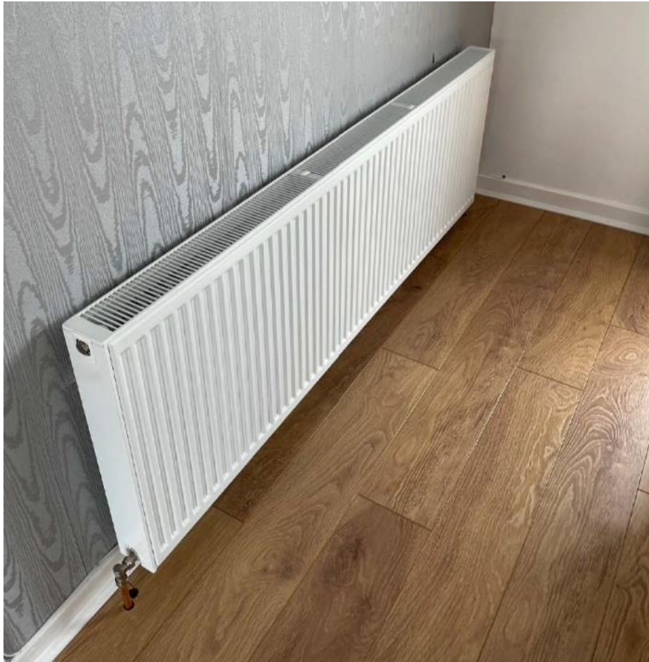
Figure 11: Example image of new radiators as supplied by the Smart Group
