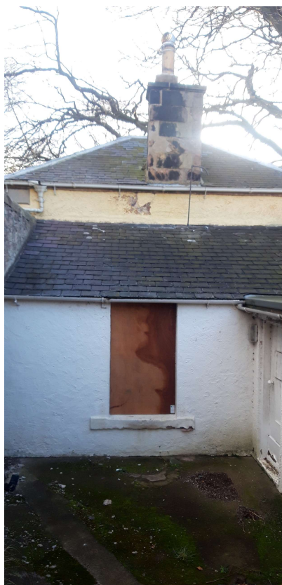
Above: Rear elevation of the bedroom and adjoining kitchen within the West courtyard
