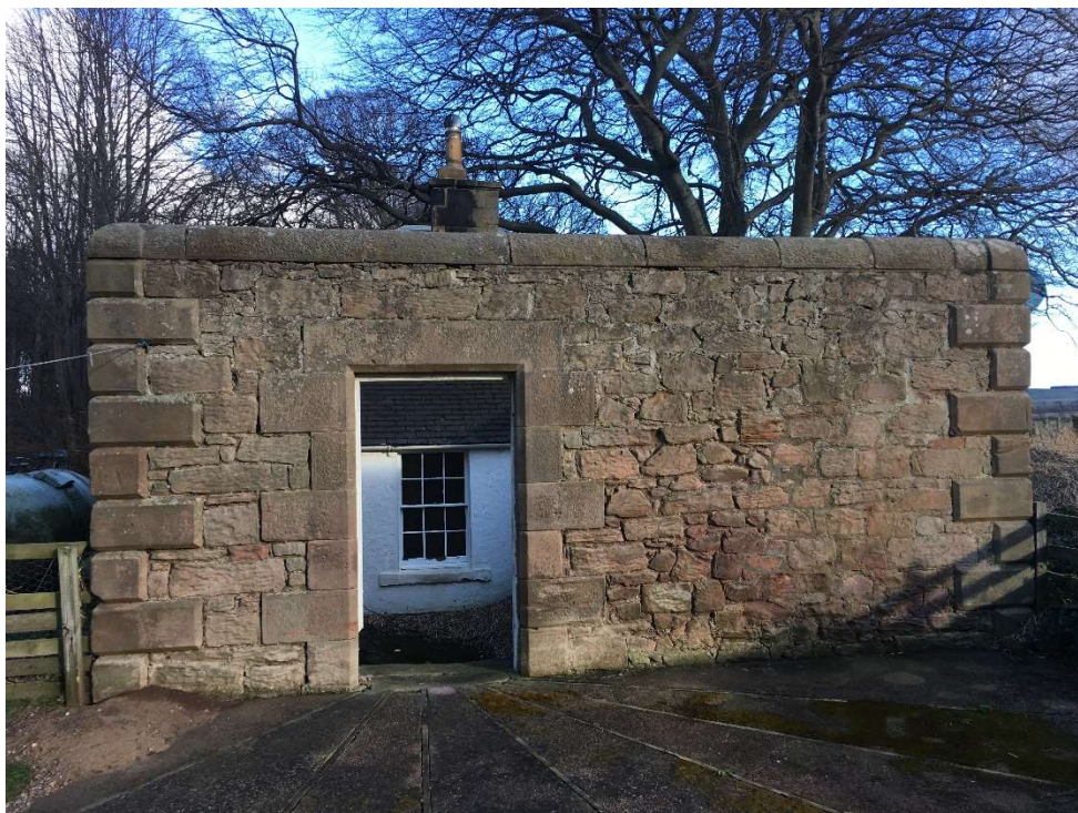
Above: Doorway to West courtyard. Note, proposal for the new window opening to the right of the doorway
