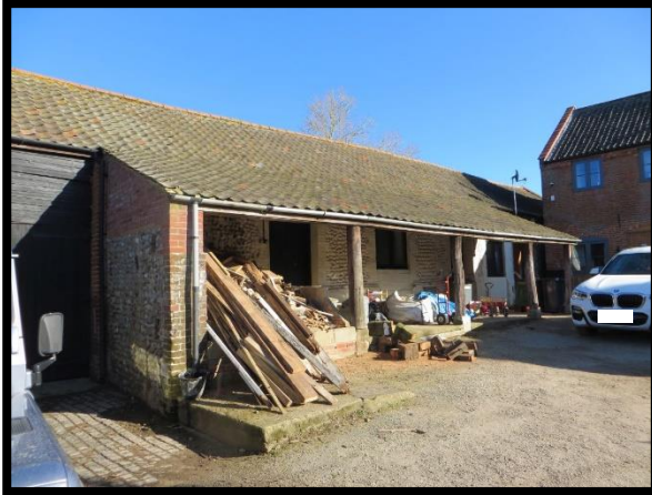
Plate 1a: Southern elevation (east)
