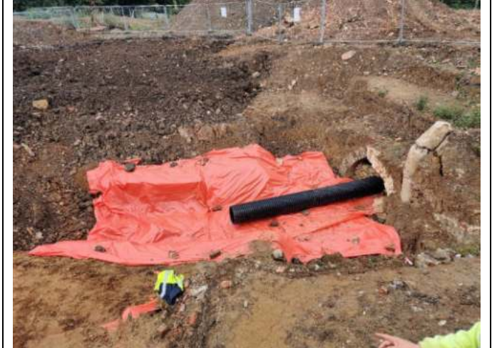
Central archaeology/culvert, installation of terram and 300mm sand and twin wall pipe as per client specification 29/09/2020
